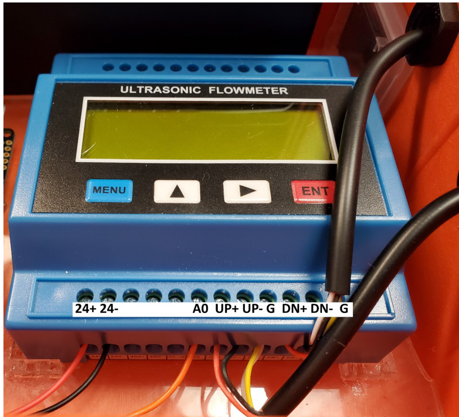
Figure 7.23 Flow meter with all wire connections. Note labels are below the ports for the wires, so in the image labels have been duplicated next to the screw terminals for clarity.
