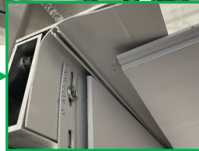
Gasketed corners to minimize leaks.
