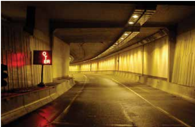
FHWA's new tunnel inspection standards require annual reports on tunnel conditions and inspection findings, such as the partially lit "DO NOT ENTER" sign in this tunnel.
