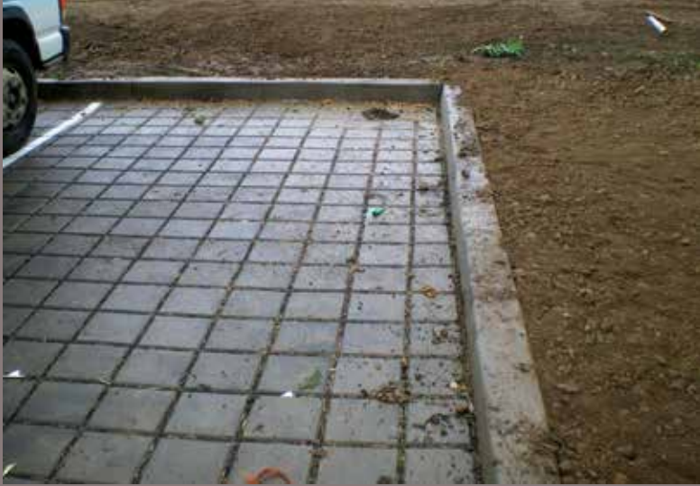
This sloping, unvegetated landscape allows the soil to wash onto the surface of the pavement and contaminate the paver joints.
