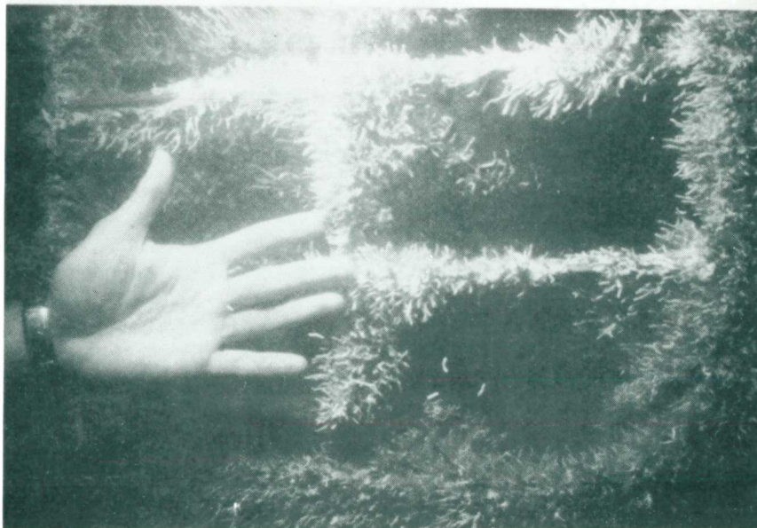
a. BEFORE CLEANING: fouling on water-intake grating
