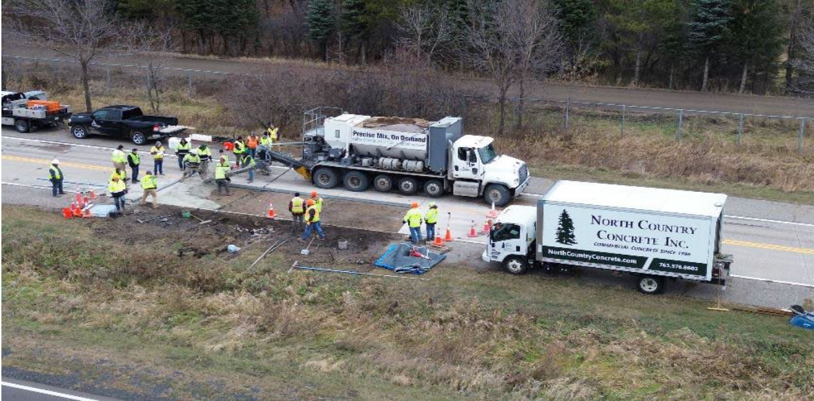
Figure 2.4. Aerial View of the pavement placement process progressing from NW to SE
