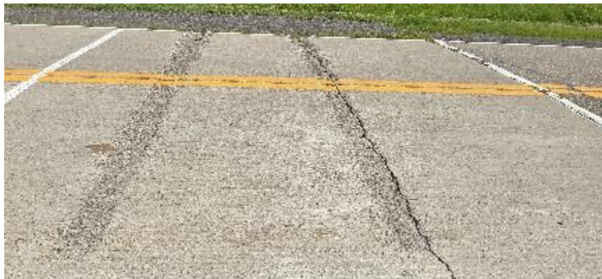
Figure 83. Transverse Ruts in PCC.
