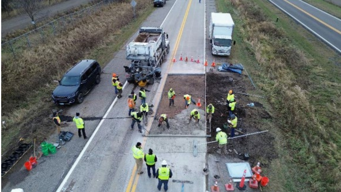
Figure 3.10 Aerial view (looking east) of the pavement placement process progressing from NW to SE showing the cables extending through the outside lane towards the cabinets. (Cabinets are not shown)
