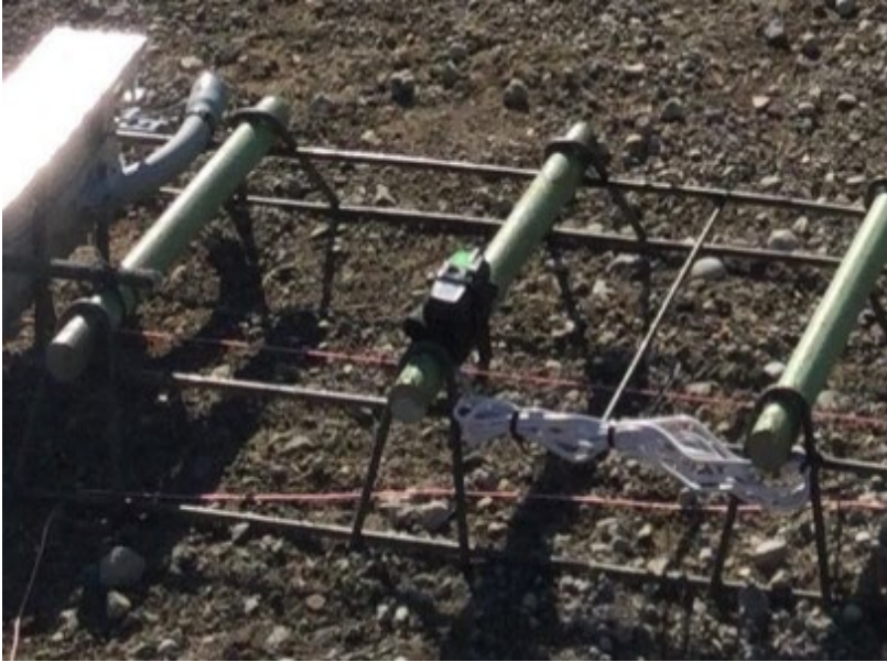
Figure 3.3 Typical Maturity Sensor Installed
