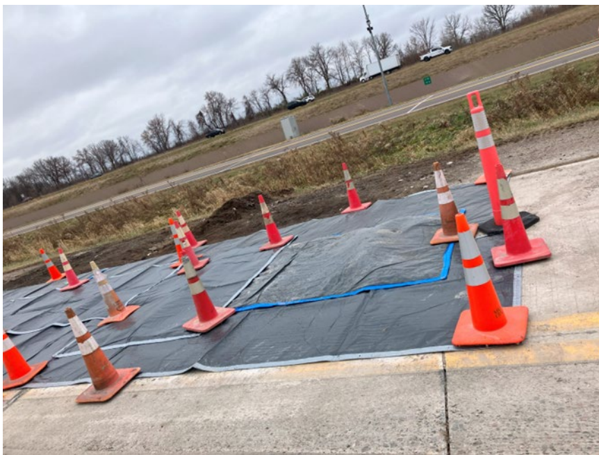
Figure 3.11 Insulative blankets were placed on the test cells after paving , finishing, texturing and applying curing compound (Alpha Methyl Styrene).
