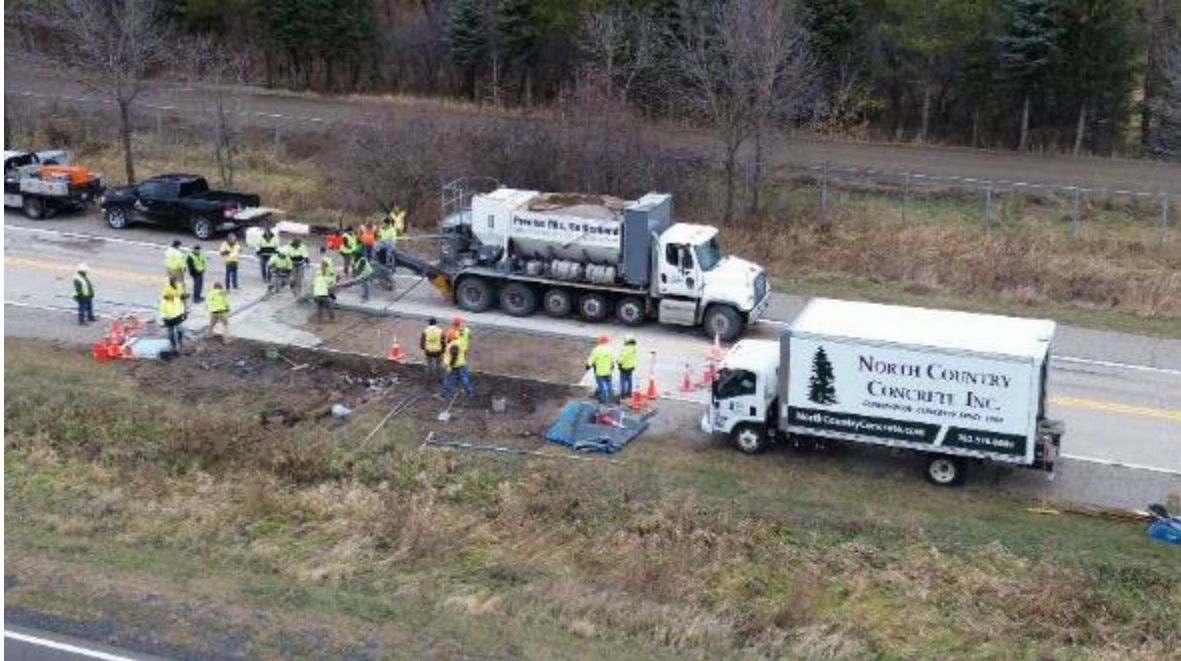
Figure 3.9 Aerial view of the pavement placement process progressing from NW to SE
