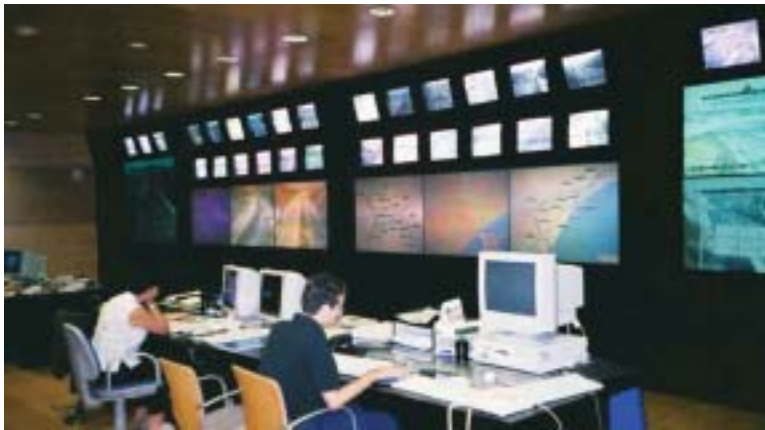
Figure 7. Traffic information center (CIVICAT) in Barcelona.
