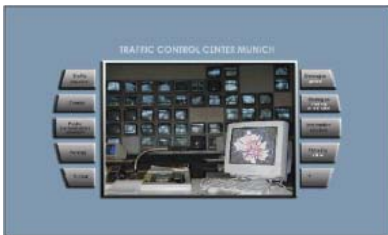
Figure 24. Traffic control center, Munich.
