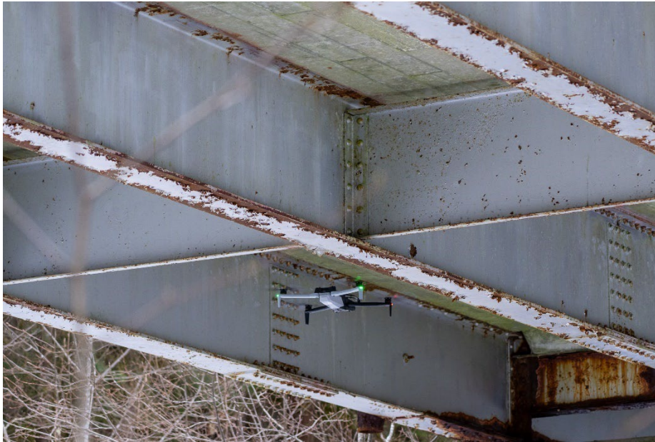
(Figure 23. Skydio X10 documentation corrosion changes during routine inspection )
