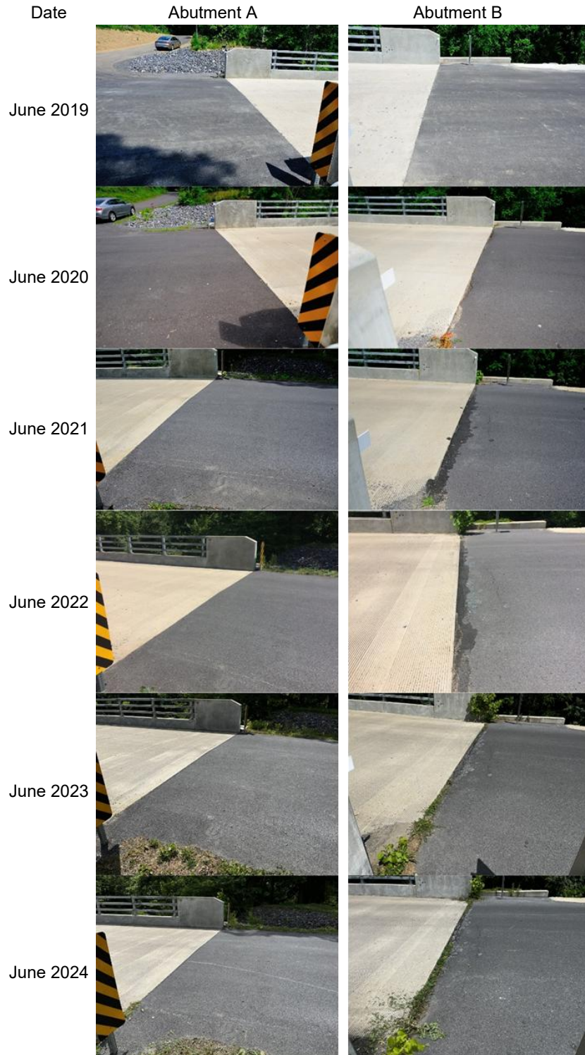
Figure 25. Photographs Comparing the Approach Condition at Abutment A (Full Integral) versus Abutment B (Semi-Integral) for Bridge 29342 No. 29342. The same roadway pavement section performed well at the stationary Abutment A while experiencing localized distress at Abutment B undergoing lateral cyclic movement in Figure 19.
