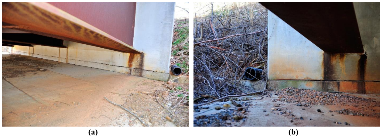
Figure 13. Photographs of Rust Staining at Full Integral Abutments: (a) Bridge 25957; (b) Bridge 25959
