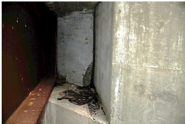
Figure 15. Photograph of Backfill Spill at Semi-Integral Abutment (Bridge 28475)
