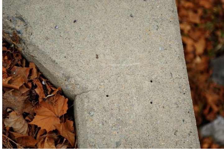
Figure 16. Photograph of Wingwall Crack at Semi-Integral Abutment with 45-Degree Skew (Bridge 28475)
