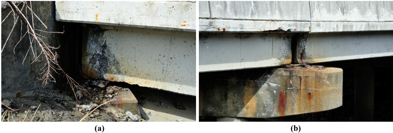
Figure 26. Photographs Showing Deteriorated Beam Ends in Bridge 4554, a Structure with Joints at Abutments and Piers: (a) Abutment A; (b) Pier 1
