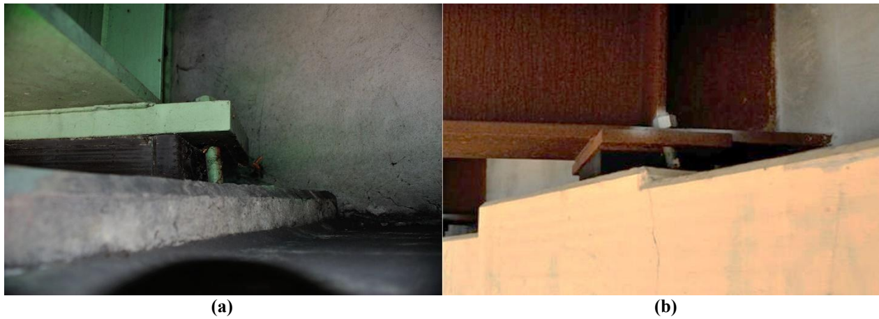
Figure 14. Photographs of Bent Anchor Bolt on Skewed Semi-Integral Abutment: (a) Bridge 20641; (b) Bridge 27544
