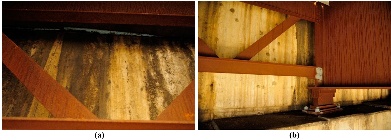
Figure 20. Photographs of Leaking Joint at Deck Extension Down the Backwalls for Bridge 27733: (a) Abutment A; (b) Abutment B
