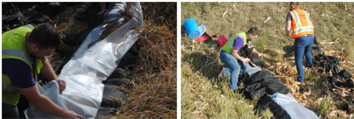
Figure 4.8 Water stop construction: sand filling and polyethylene sheet folding (left); interlocking with treatment bags with water stop between layers (right).
