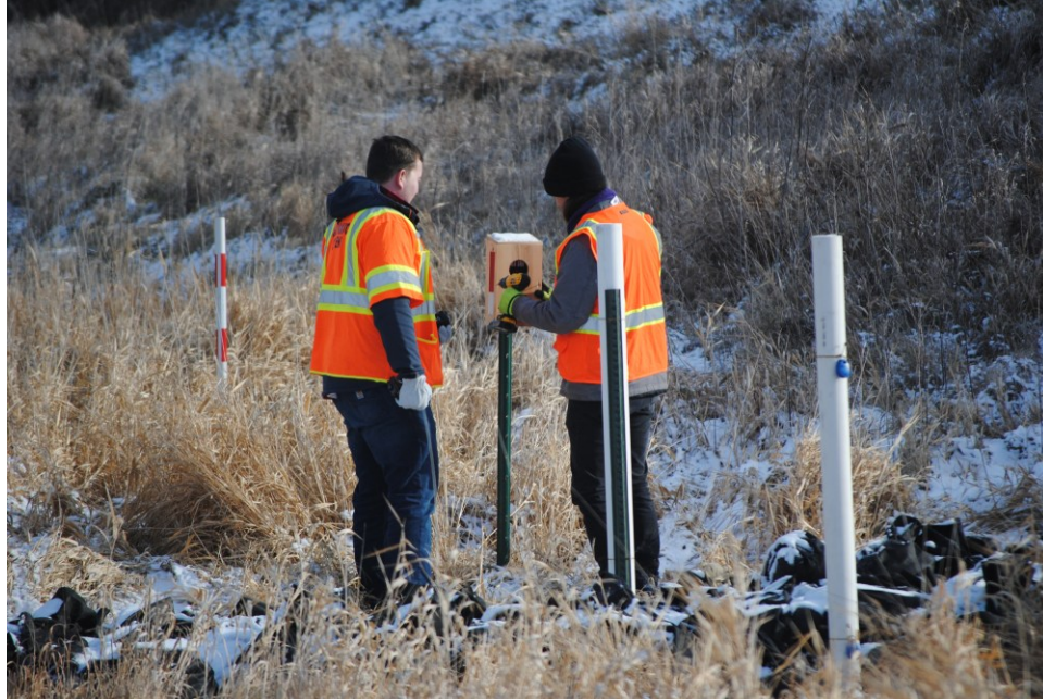
Figure 4.9 Instrumentation installation December 3, 2024. From left to right along ditch line: snowmobile warning post with reflective tape, time lapse camera being installed in an imitation “bird house” on post, post and PVC standpipe for ditch water access up
