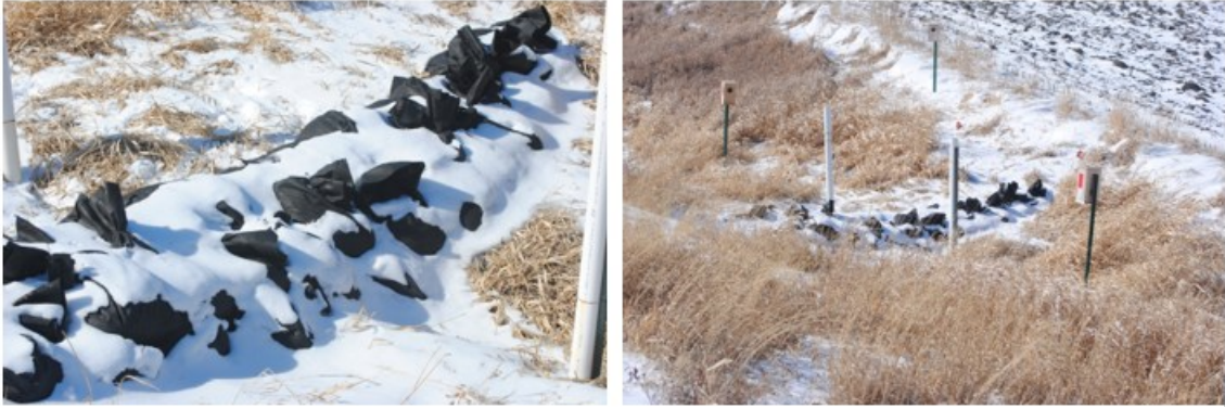
Figure 4.11 Berm as installed at Sterling North (views upstream and to west). February 21, 2025.
