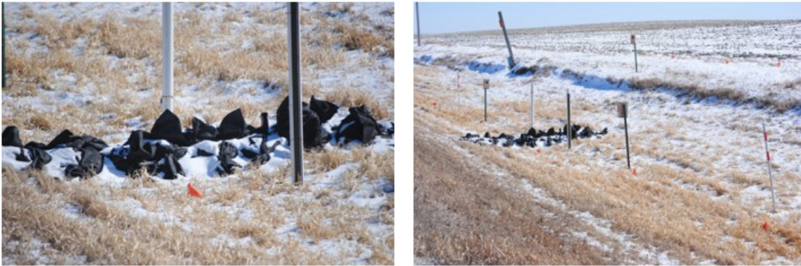
Figure 4.13 Berm as installed at Willow Creek East (views upstream and to east). February 21, 2025.
