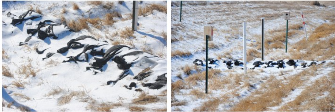
Figure 4.12 Berm as installed at Willow Creek West (views upstream and to west). February 21, 2025.
