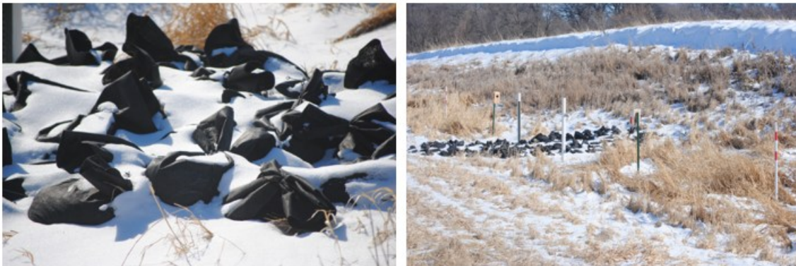
Figure 4.10 Berm as installed at Sterling South (views downstream and to east). February 21, 2025.
