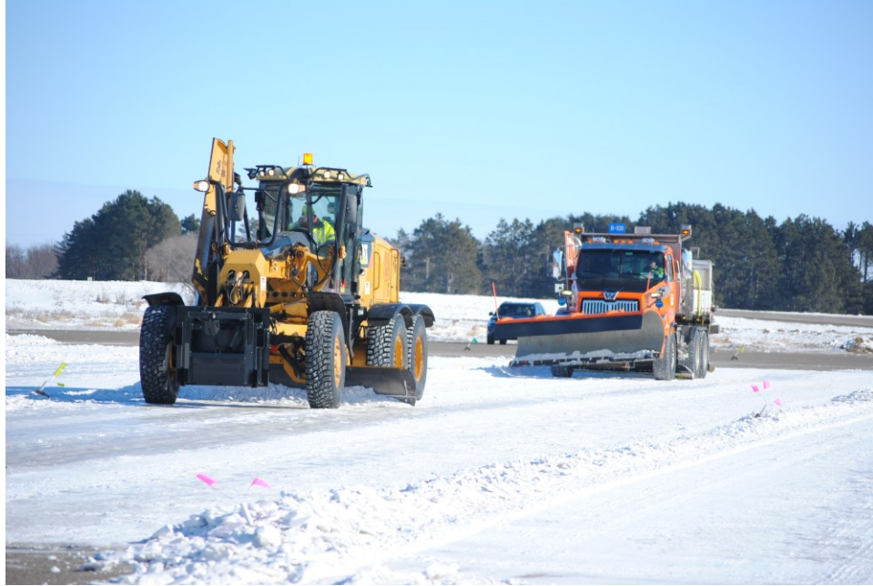
Figure 4. Motor grader and plow truck using underbody plow to cut and shape lanes at the skid pad prior to testing.
