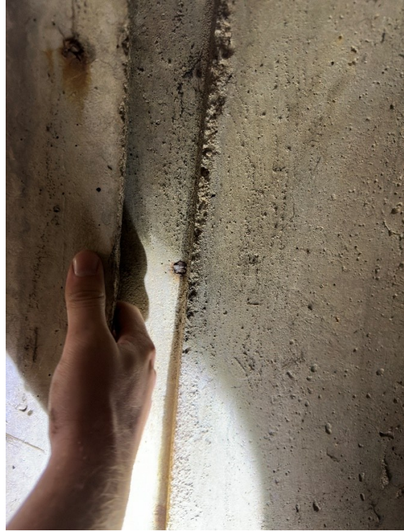
(b) Culvert 2251023, District 8: 3 in. separation at first joint
