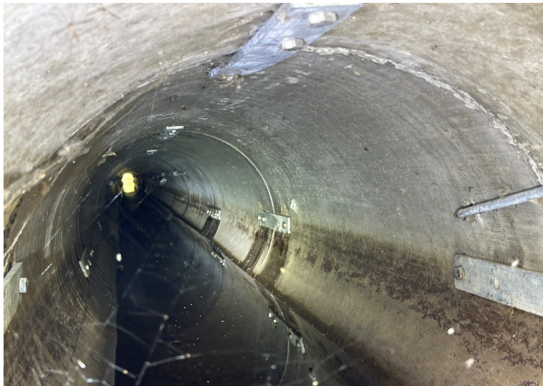
(c) Culvert 2181739 in District 3, combination of flat bar ties and interior ties
