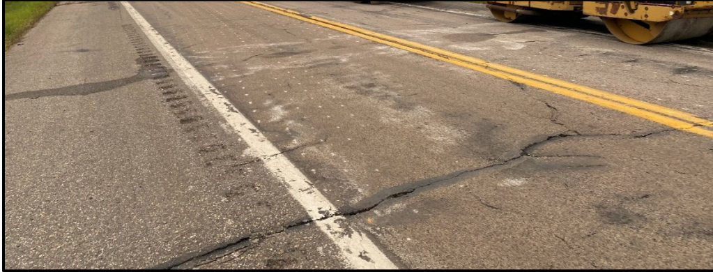
Figure B 1: CSAH 15 pavement condition prior to construction
