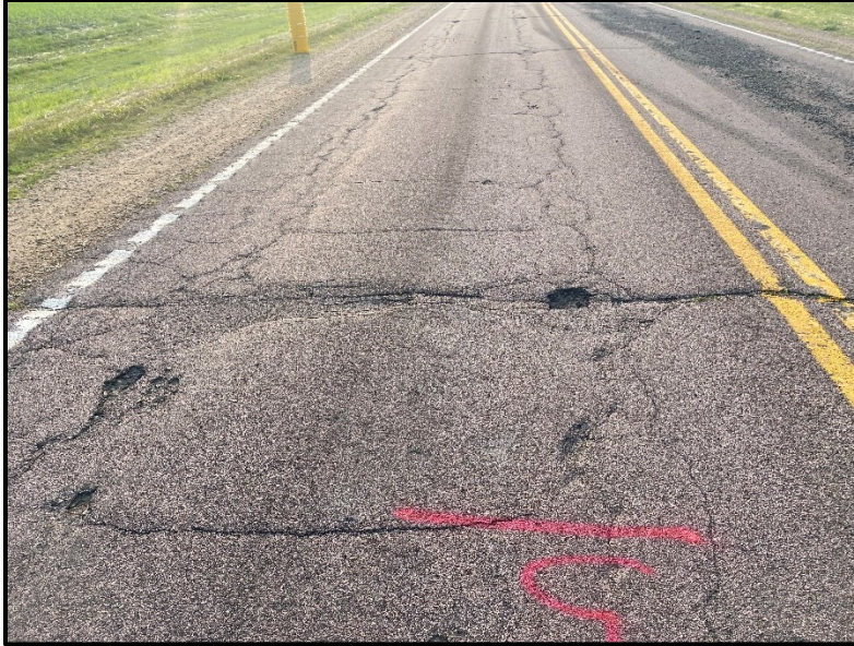
Figure B 18: CSAH 24 pavement condition prior to construction
