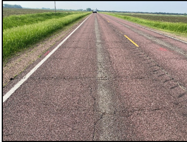
Figure B 6: CSAH 11 pavement condition prior to construction
