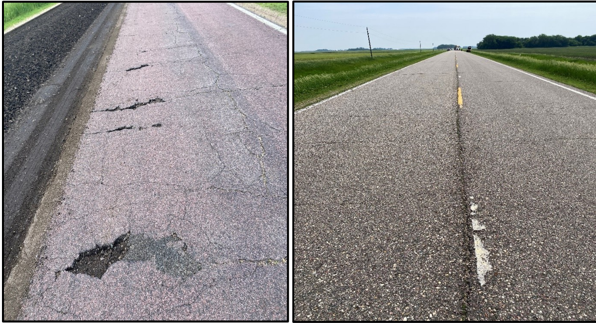
Figure B 11: CSAH 20 pavement condition prior to construction
