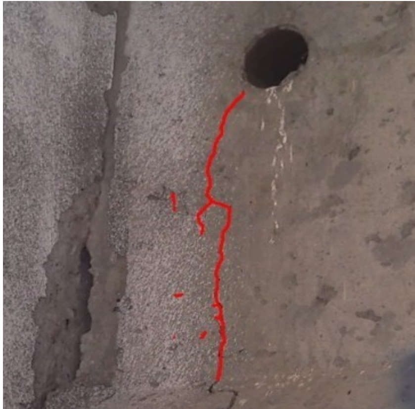
FIGURE 23 Virtual Crack Visualization Overlaid on Bridge Surface Defect Image Based on CV Server Calculations
