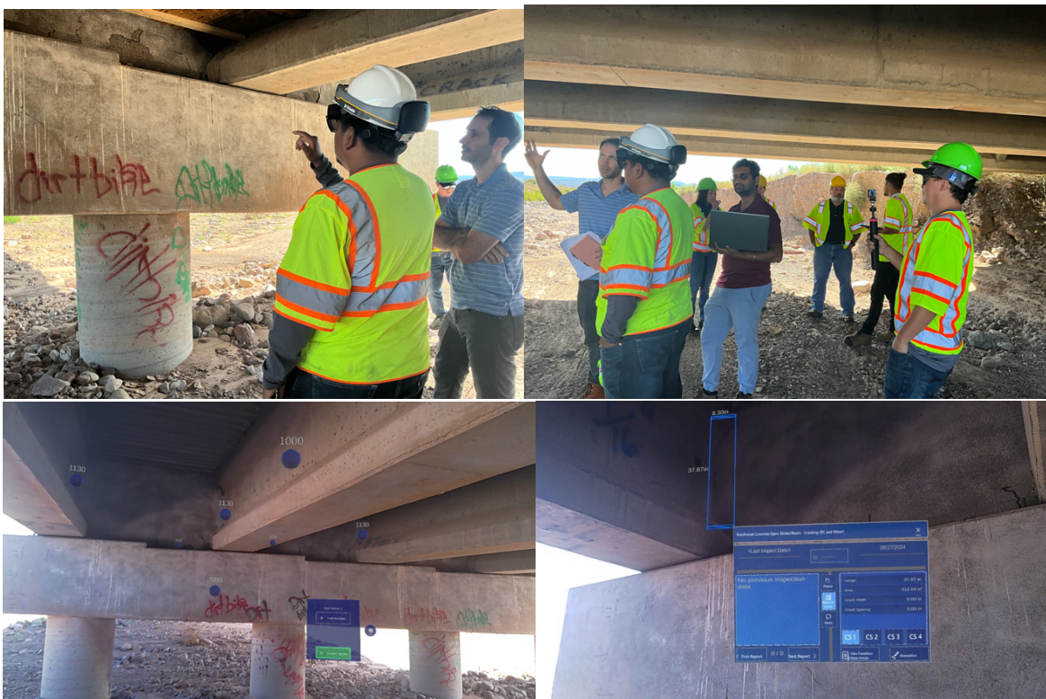
FIGURE 28 Photos of Stakeholders working with the AR App at Socorro bridge (top), along with first person AR-view of noted defects (middle), and crack measurement panel (bottom)
