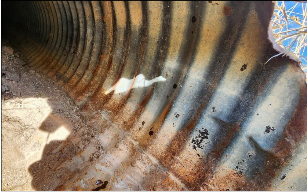
FIGURE 101: Considerable amount of corrosion on the inside of the culvert on US 60 MP 204.33.
