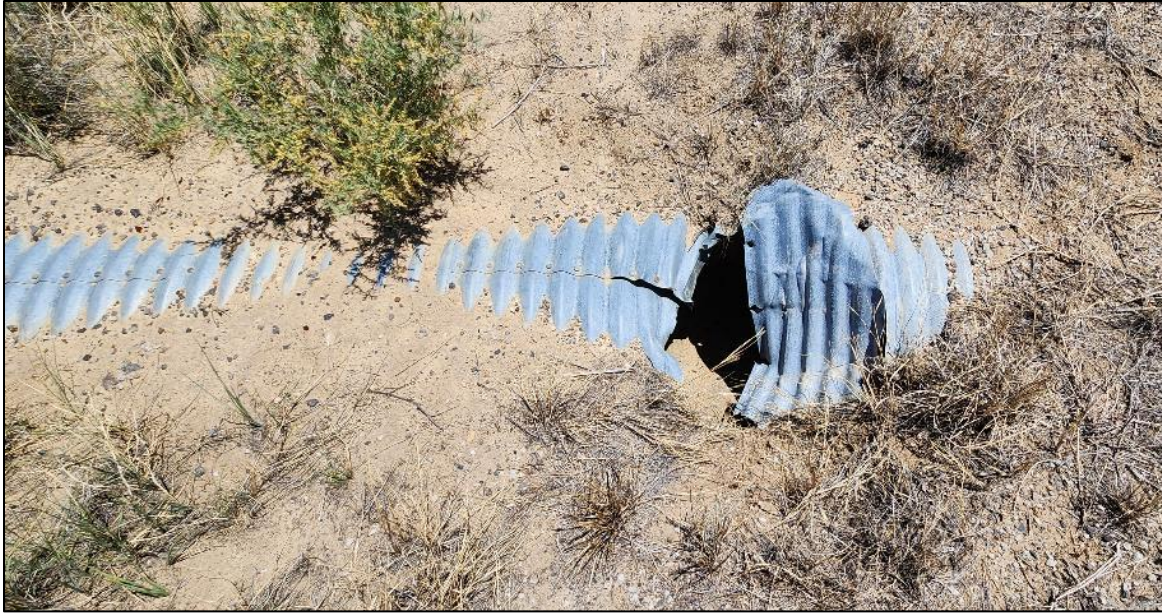
FIGURE 66: Outlet of culvert on NM 117 MP 55.8 showing collapsed location.
