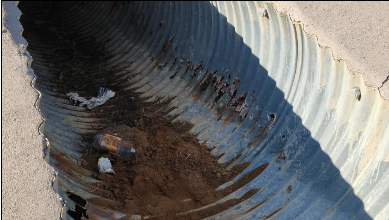
FIGURE 35: Culvert I-40 MP B showing the extent of corrosion roughly 1/3 up the side of the culvert.
