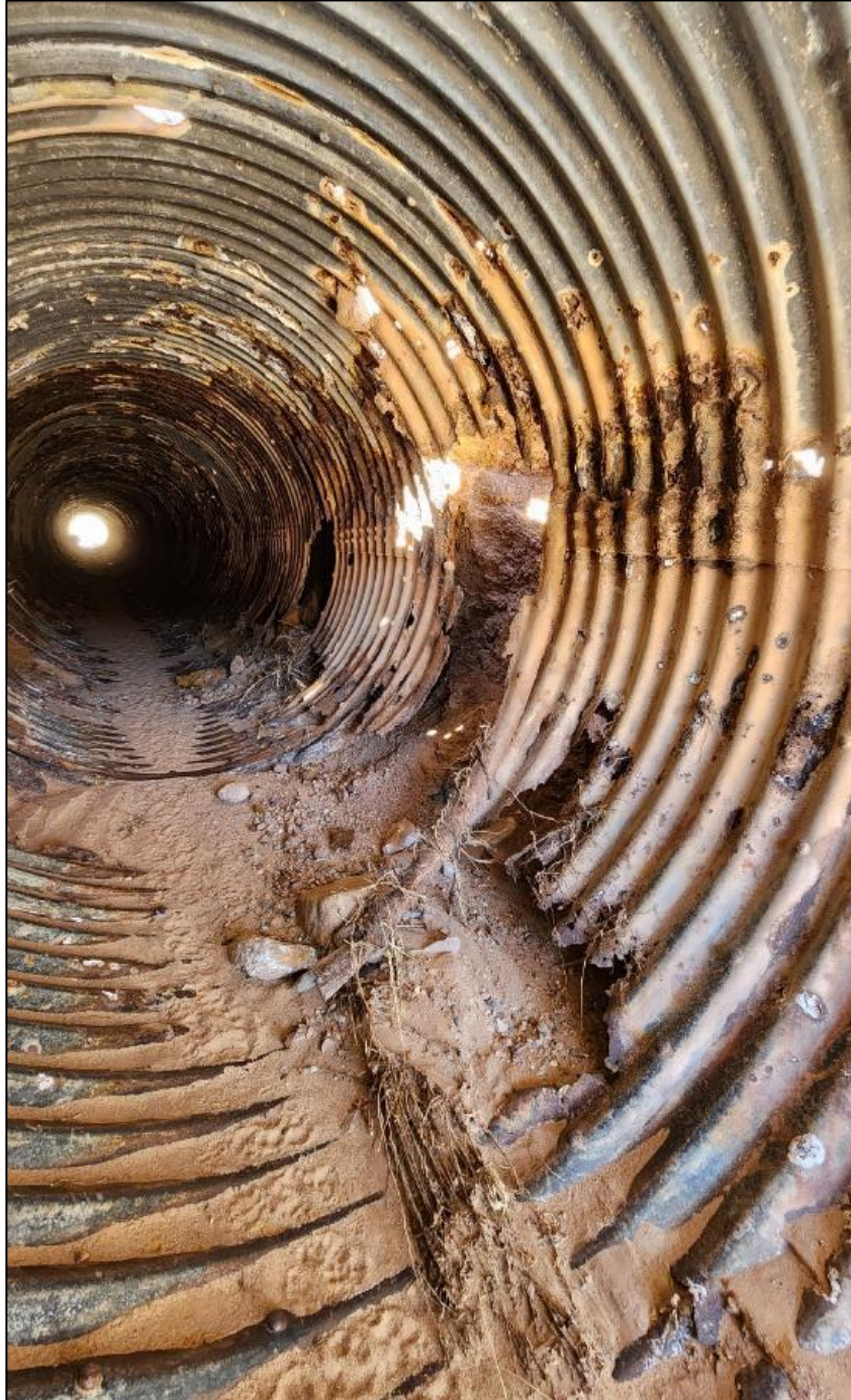
FIGURE 87: Culvert on NM 290 MP0.65, outlet side, approximately 10 feet in from end. Extreme corrosion with backfill being undermined during last flow event.
