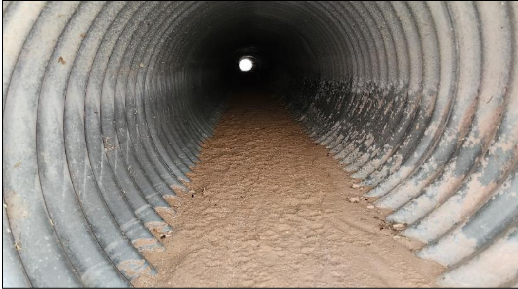
FIGURE 95: No corrosion present on the inside of the culvert on NM 290 MP 1.0.
