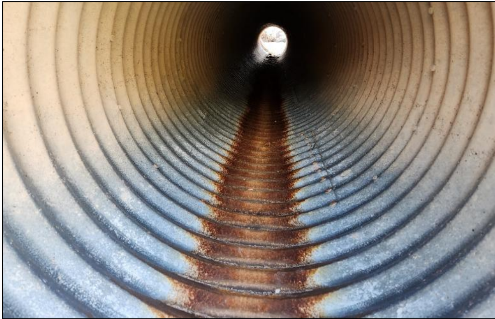
FIGURE 6: Inside of the outlet side of the culvert on I-25 (NB) MP 107.86.
