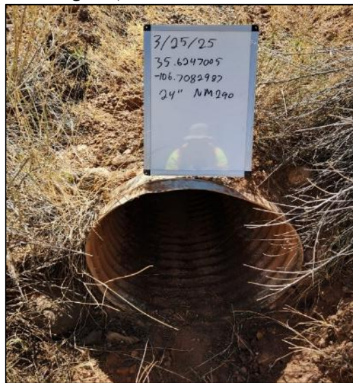
FIGURE 90: Inlet of culvert on NM 290 MP 0.91.
