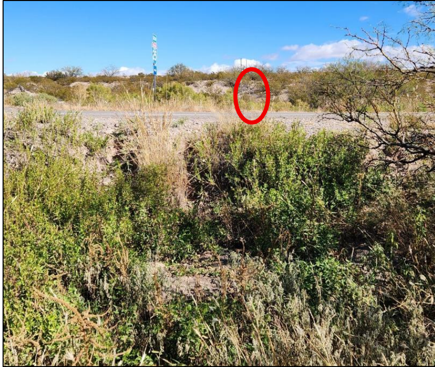
FIGURE 80: Approximate inlet side of culvert on NM 181 MP 5.48, buried in dirt. Culvert road warning marker circled in red.
