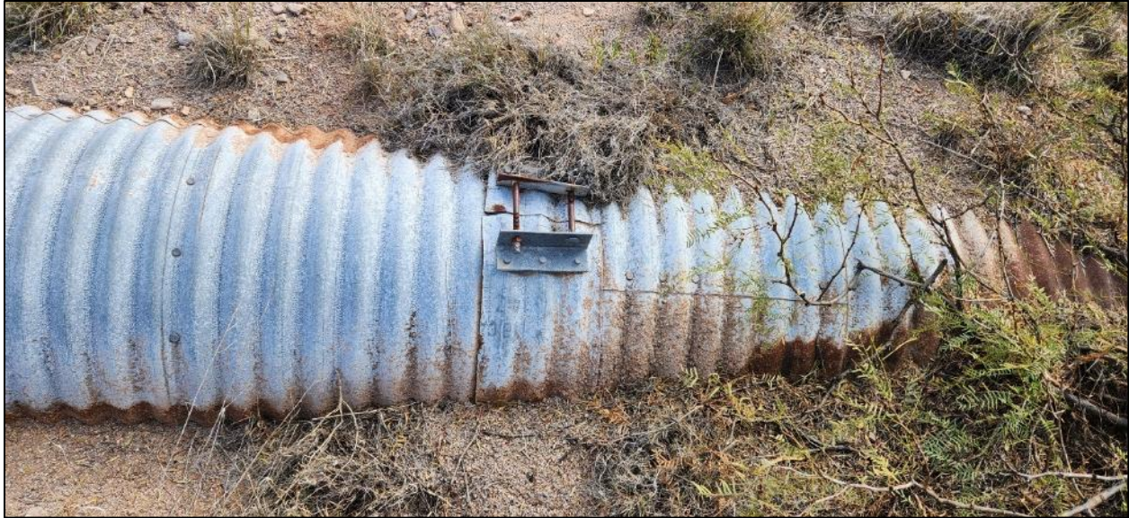
FIGURE 7: Outside of the outlet side of the culvert on I-25 (NB) MP 107.86.
