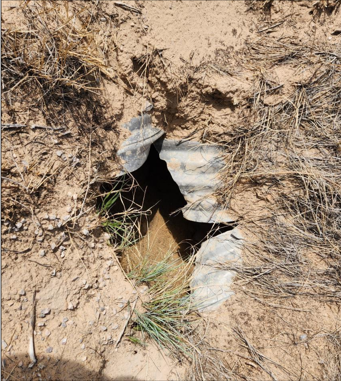
FIGURE 61: Close-up of collapsed culvert, roughly 3' by 2', NM 117 MP 55 culvert.
