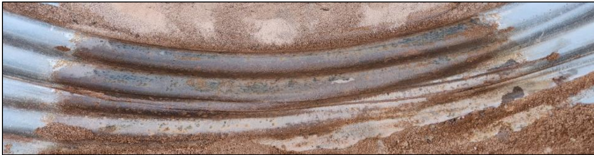
FIGURE 23: Slight corrosion on the bottom of the culvert underneath the sandy soil present on I-25 MP 264.2.
