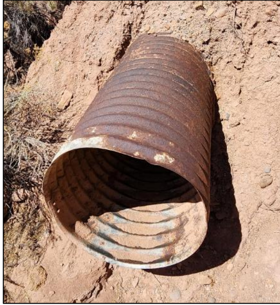
FIGURE 92: Culvert on NM 290 MP 0.91, outlet side with excessive outside corrosion.
