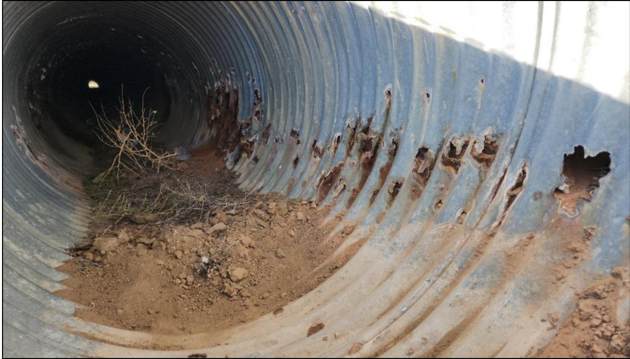
FIGURE 34: Culvert I-40 MP 121 A showing the extent of corrosion roughly 1/3 up the side of the culvert.
