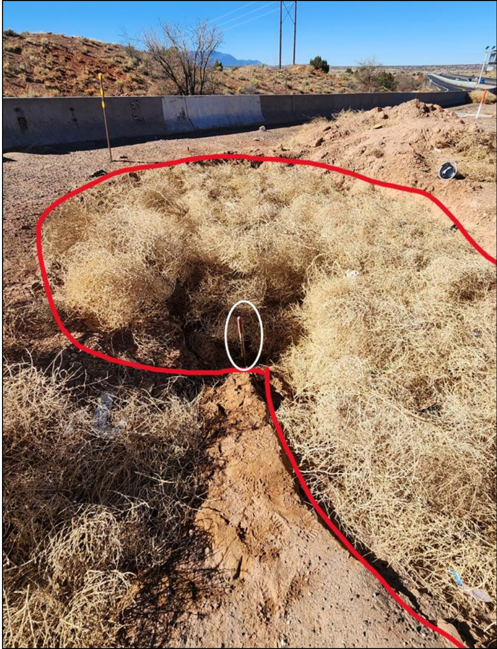
FIGURE 19: Image of the tumbleweed-filled “Hole,” outlined in red, and a 5’ 6” long shovel outlined in white from culvert between Exit 264 offramp and I-25.
