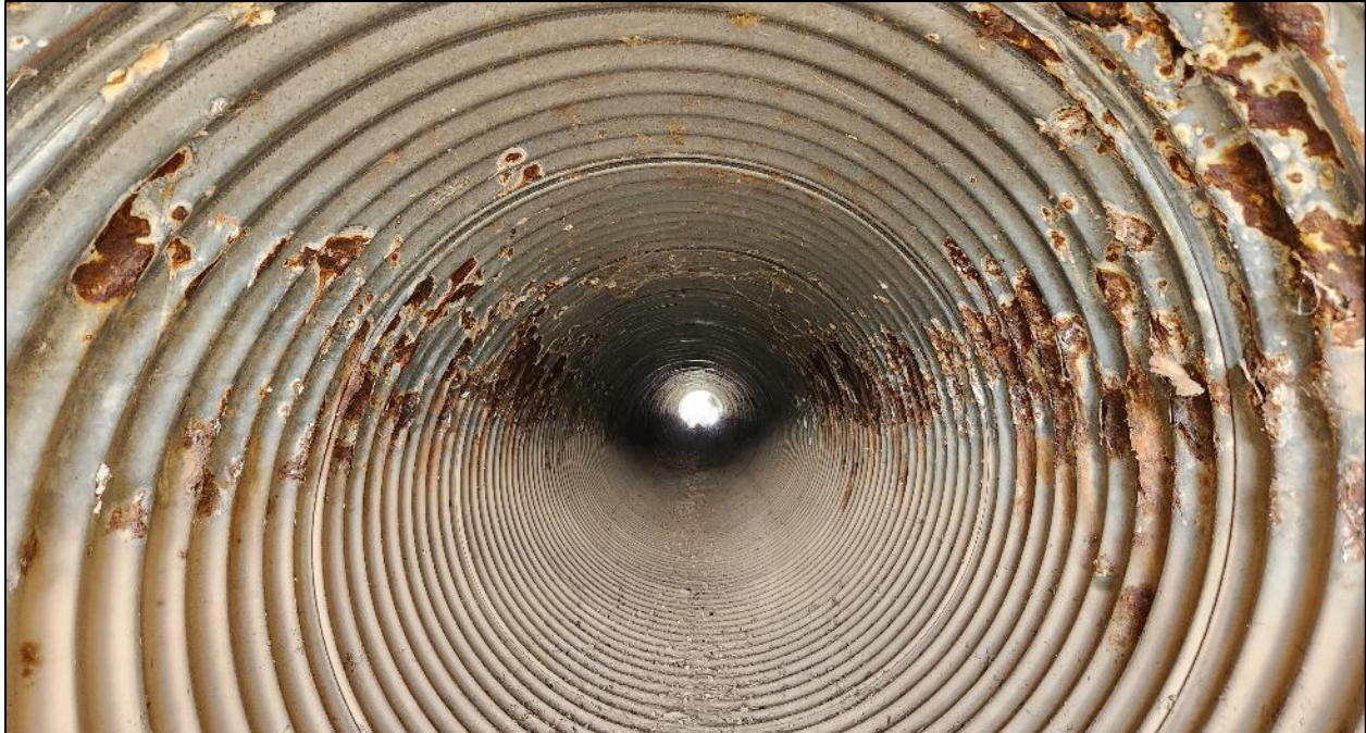
FIGURE 72: Culvert on NM 117 MP 57, inlet side, significant corrosion on the upper half of the culvert and minimal to no corrosion on the lower half.
