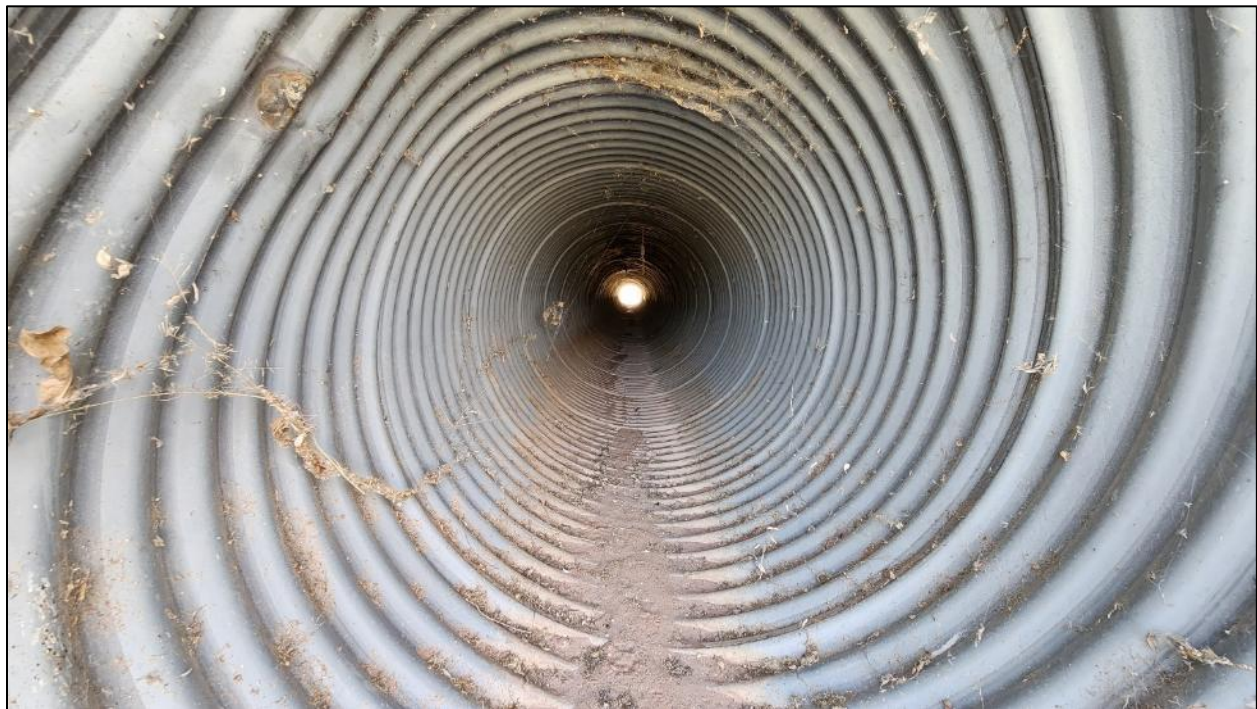
FIGURE 76: Eastern 36" culvert on NM 128 MP 21.93 facing south at inlet.
