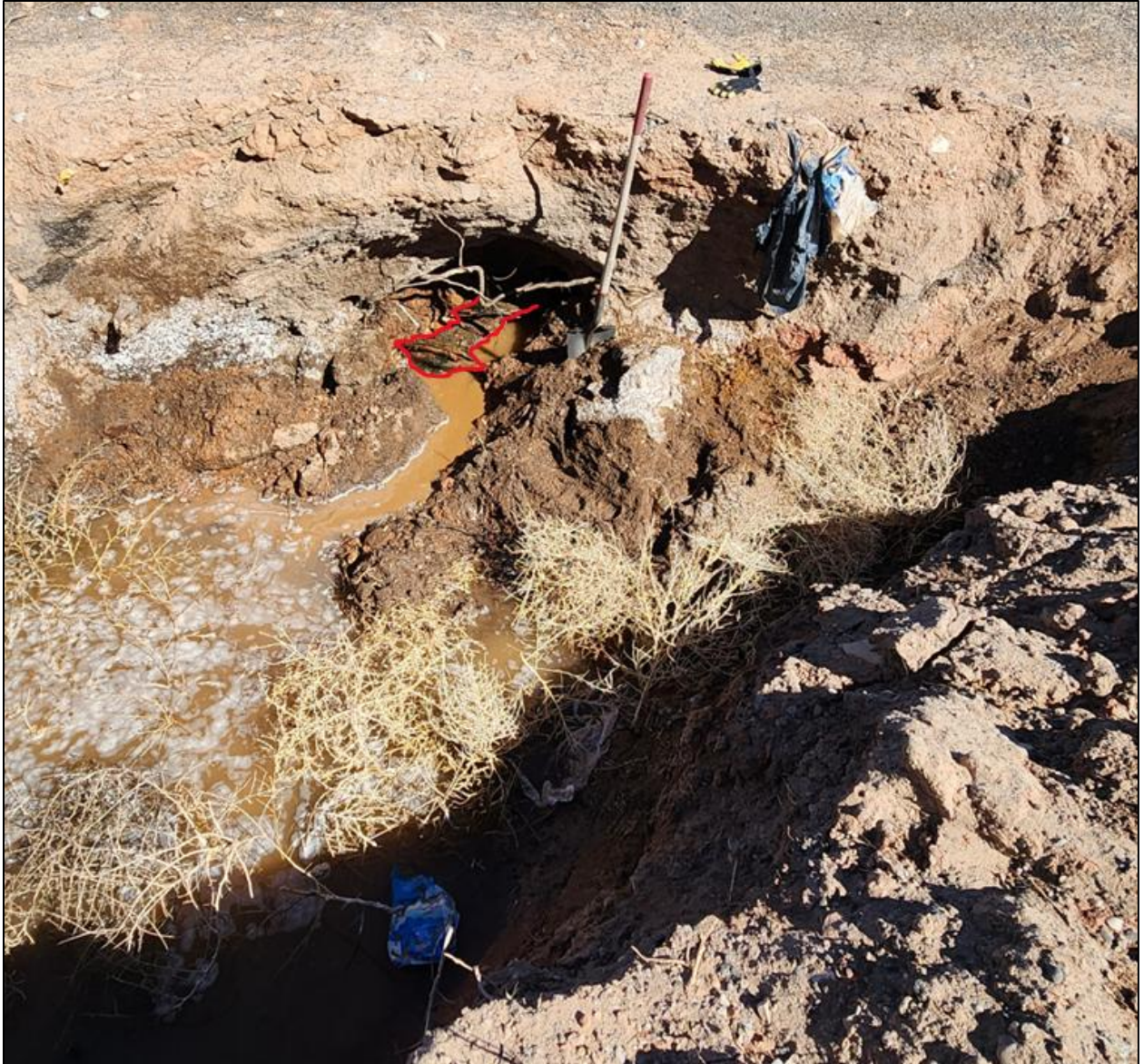
FIGURE 20: Image of 24" (estimated) outlet with a red line highlighting the only metal remaining of culvert between Exit 264 offramp and I-25.
