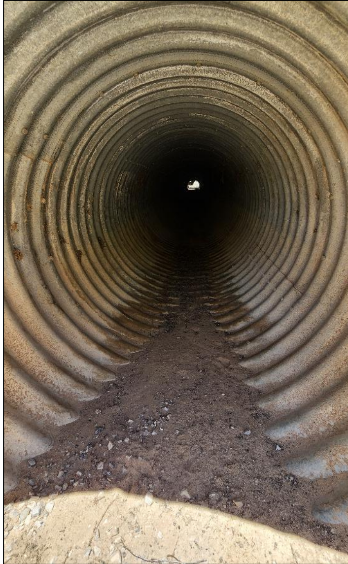
FIGURE 65: Inside of the inlet side of the culvert on NM 117 MP 55.8, indicating some slight corrosion on the bottom inside of the culvert.
