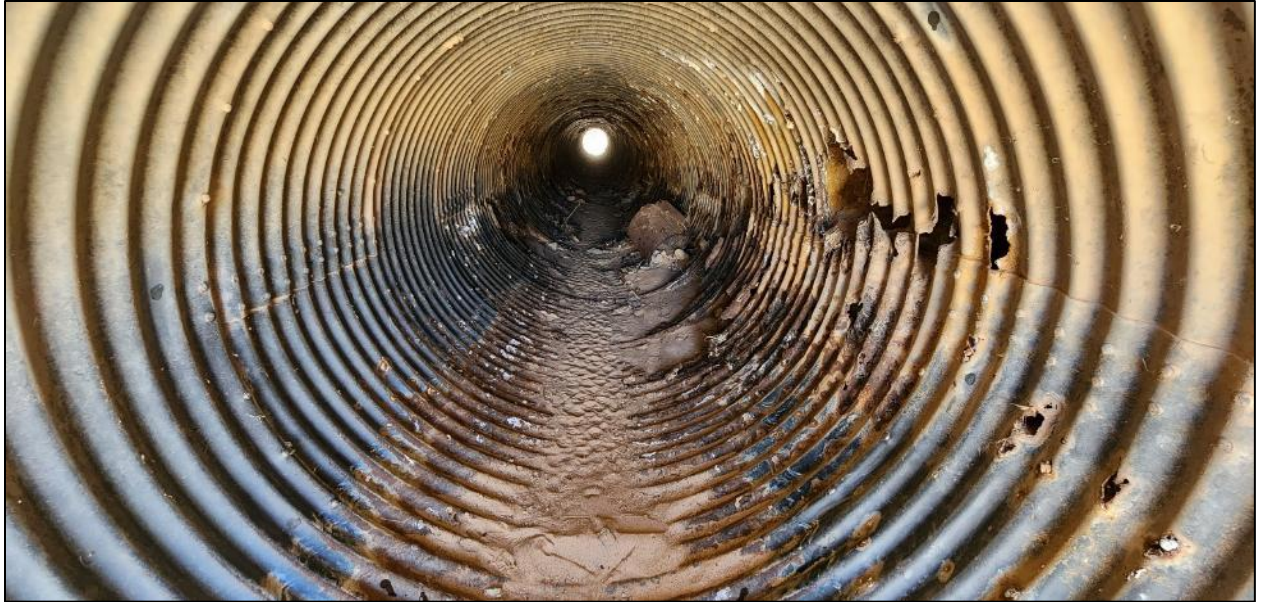
FIGURE 85: Culvert on NM 290 MP0.65, inlet side, approximately 10 feet in from the end. Image shows multiple large sections of the culvert's bottom missing in addition to a large hole halfway up the right side.
