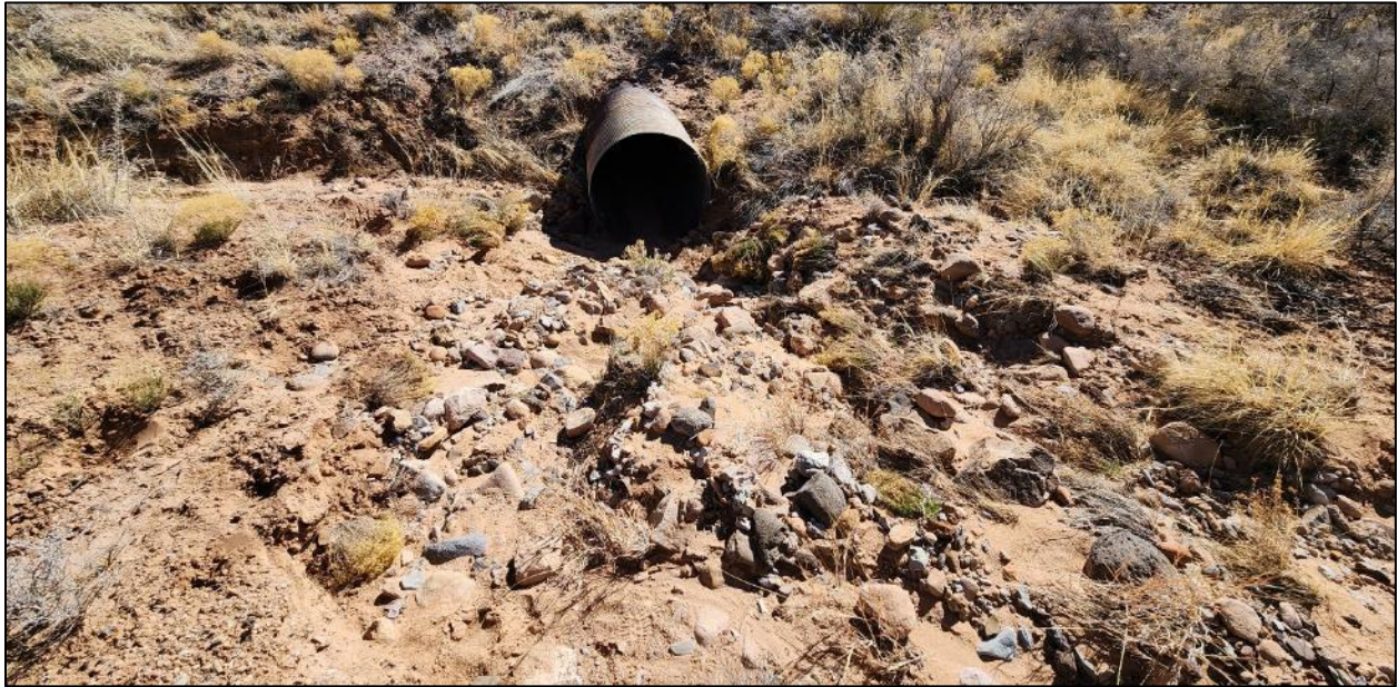
FIGURE 89: Culvert on NM 290 MP 0.65, inlet side. Image of the rocky ground around the inlet of the culvert.
