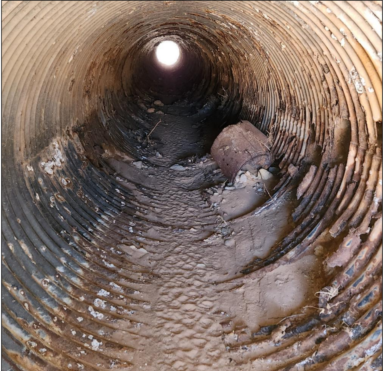
FIGURE 86: Culvert on NM 290 MP 0.65, inlet side, approximately 10 feet in from end. Image shows a zoomed-in view of the culvert's bottom where large sections are missing and what appears to be an old, metal bucket stuck in one of the corroded holes.
