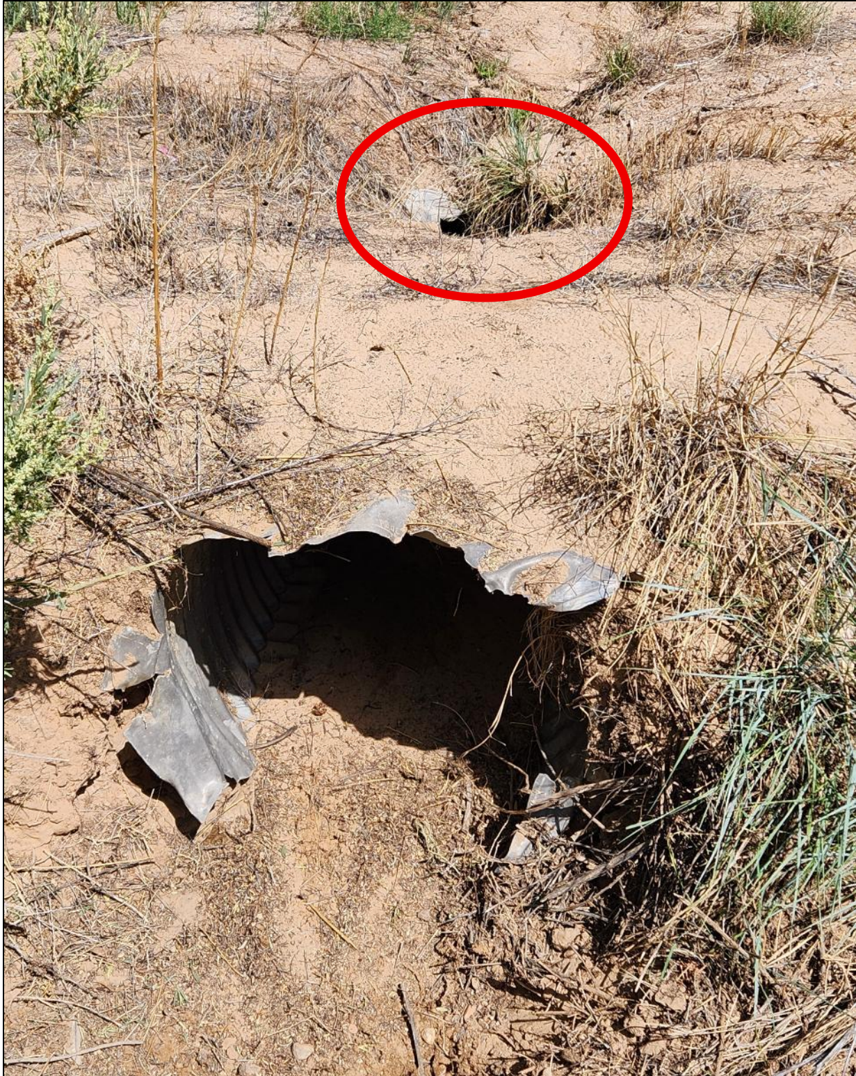
FIGURE 60: Inlet side after removal of brush with collapsed section of the culvert circled in red, NM 117 MP 55 culvert.
