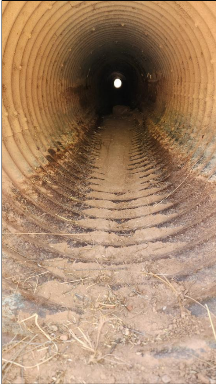
FIGURE 91: Culvert on NM 290 MP 0.91, inlet side showing corrosion on the inside bottom.
