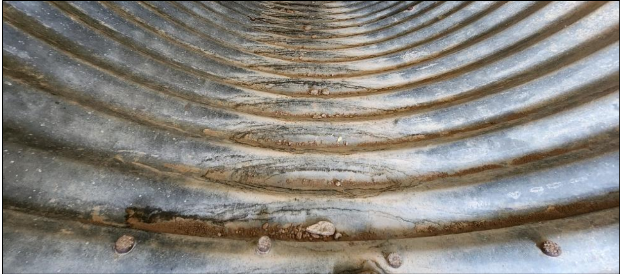
FIGURE 98: No corrosion was present on the inside of the culvert on US 60 MP 203.41.
