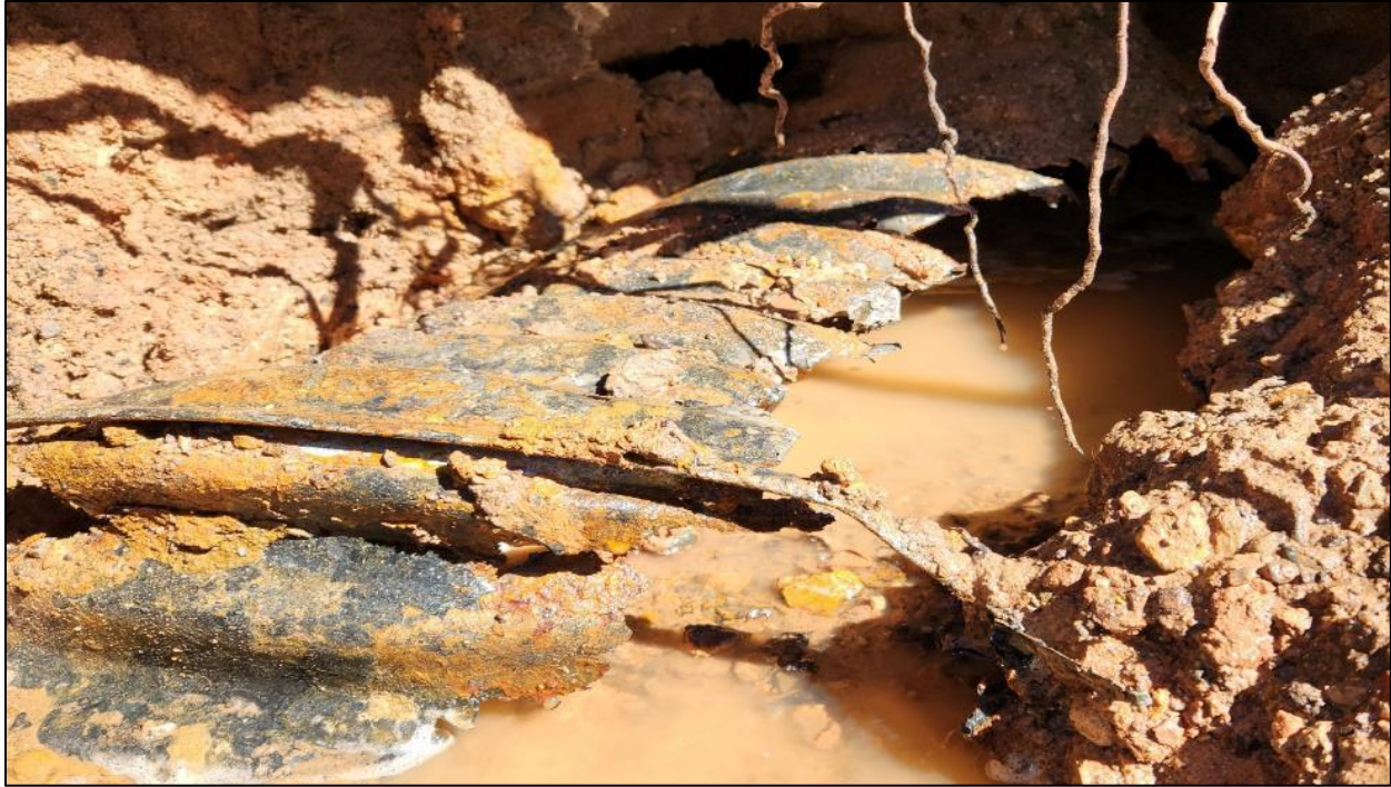
FIGURE 21: Close-up image of the near fully corroded second culvert outlet from culvert between Exit 264 offramp and I-25.
