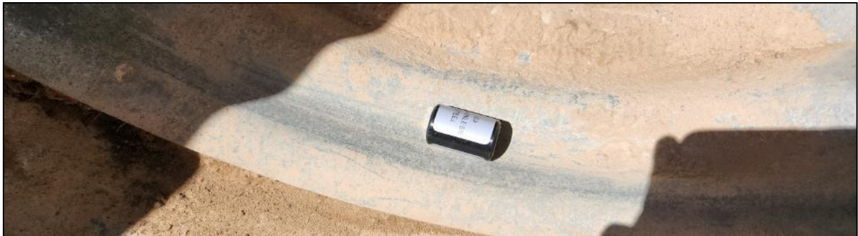
FIGURE 28: No corrosion was present on the inside of the I-25 (SB) MP 278.7 culvert.
