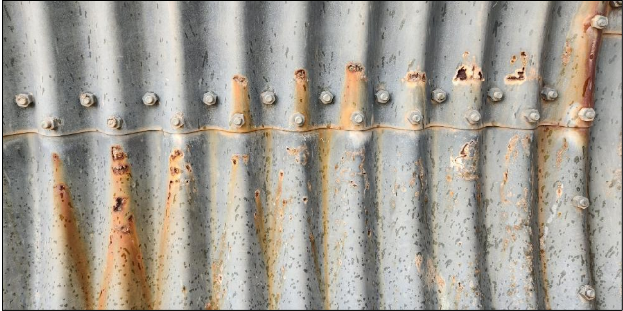
FIGURE 11: Inside wall of the outlet side of the culvert on I-25 MP 113.04.
