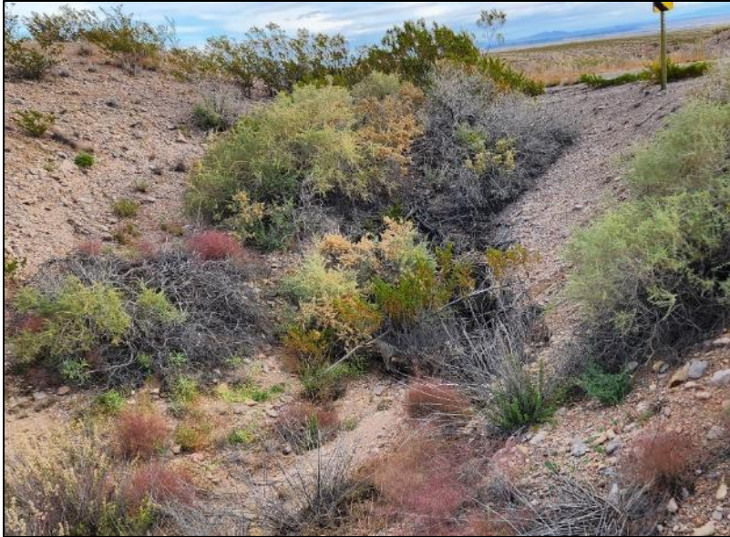
FIGURE 39: Approximate location of culvert on NM 1 MP 20.61, buried in thick brush.
