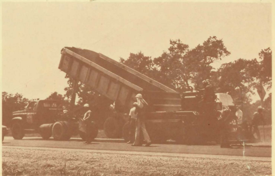
Standard construction equipment is used to pave with Sulphlex as shown at the field test section on Loop 1604 north of San Antonio, Tex.
