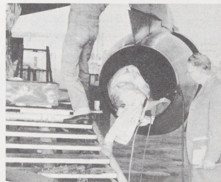
Maint. Insp. Rich Melberg at WAL observing crack weld repair of thrust reverse clam shell on Boeing 720 at LAX
