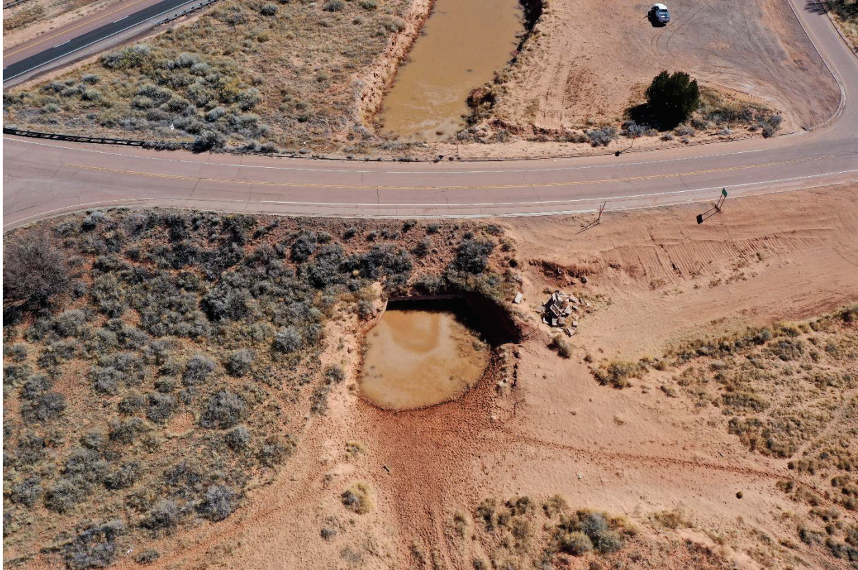
Figure 1 – An example of a maintenance problem area, where ponding and erosion are evident.
