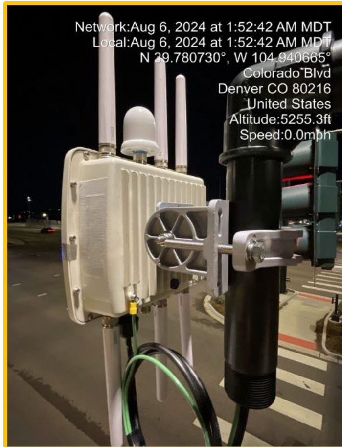
Figure 18: Photo of an installed RSU at an intersection in Denver, Colorado
