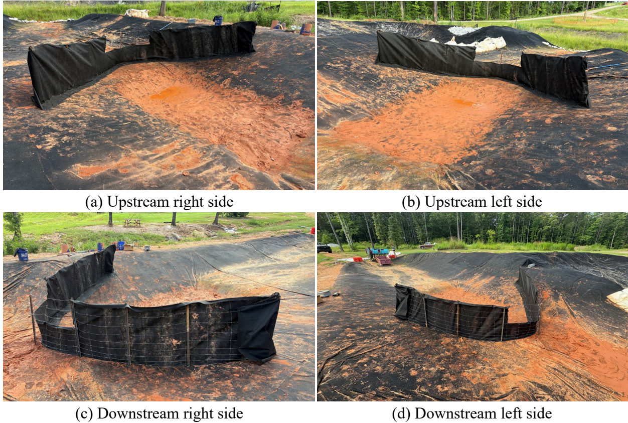
Figure 4.4: Modified Silt Fence
