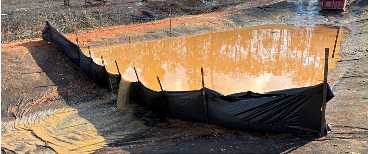
Figure 4.28: Installation 5 After Test C
