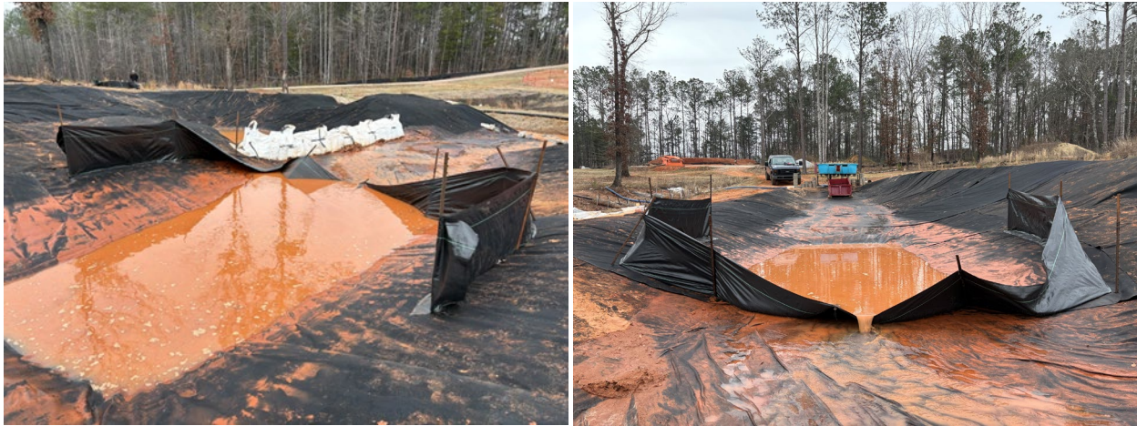
(a) Failure, facing downstream
