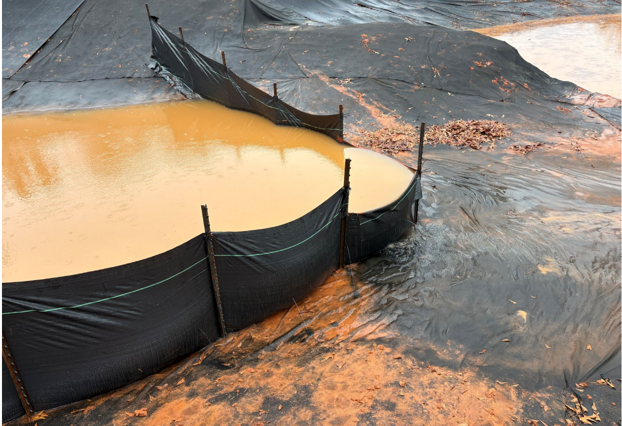
Figure 4.25: Installation 3 After Test C
