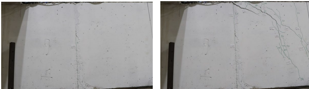
(a) Crack at cold joint under self-weight
