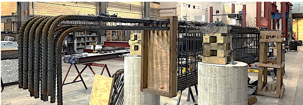
Figure 5-15 Steel cage of III-1.85-00-V and III-1.85-00-V-R with wooden stopper in between the interior and the exterior section
