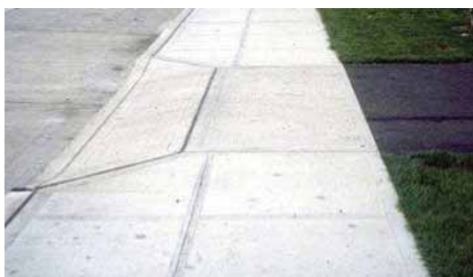
Driveways should be designed so that the sidewalk continues through the driveway in a relatively flat and level alignment.
