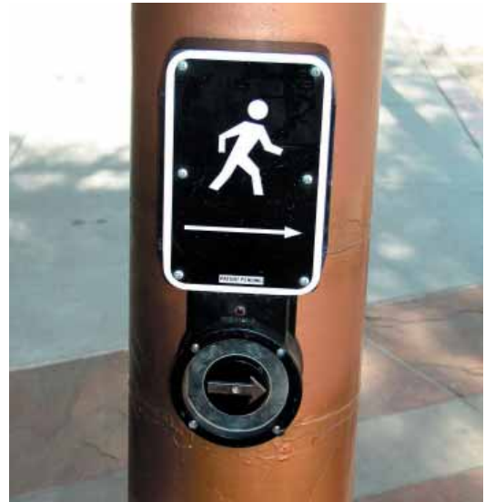
Push buttons such as this one should be placed where they can be easily accessed when waiting to cross an intersection.
