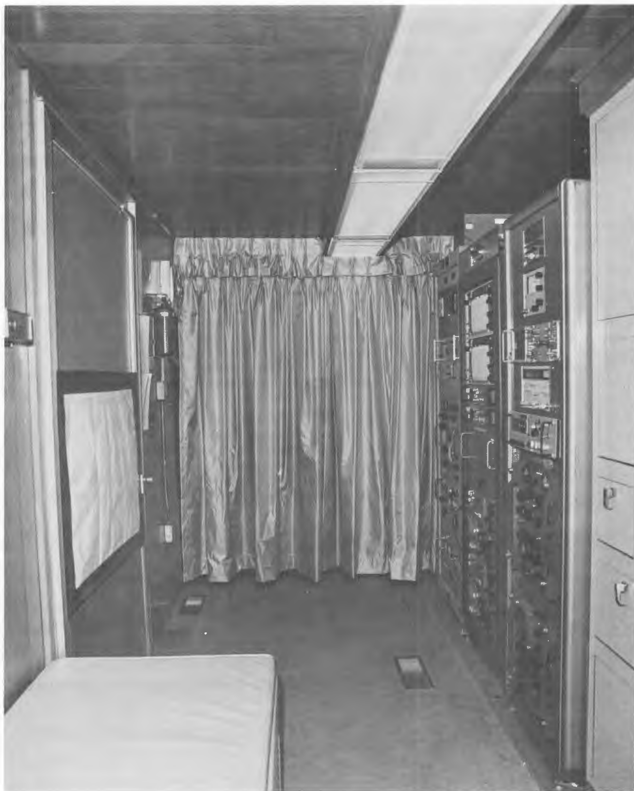
FIGURE 4. INTERIOR OF ELECTRONICS VAN SHOWING EQUIPMENT RACKS
