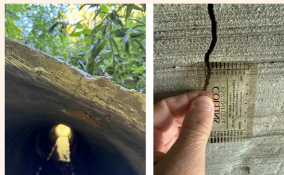
Cracks in Conventional Cementitious Liners
