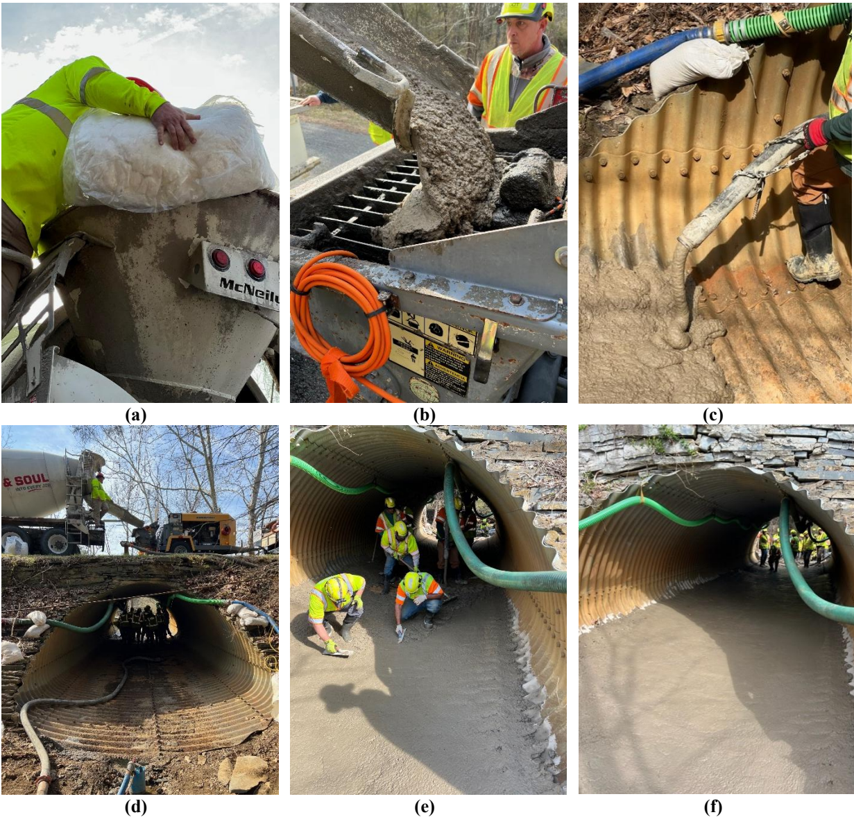
Figure 9. Photographs of Field Test: (a) Polyethylene Fiber Added on Site; (b) ECC Delivered to the Pump; (c) ECC Delivered in the Culvert Invert; (d) Culvert at the Beginning of Placement; (e) VDOT Crew Placing ECC in the Invert; (f) Placement Finished. ECC = engineered cementitious composite.
