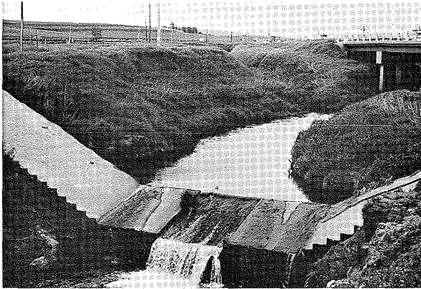
Plate 9. Grade stabilization structure consisting of double row of steel sheetpile with a concrete core and cap. Note large crack in right side resulting from adjacent landslide caused by downstream scour in plunge pool.
