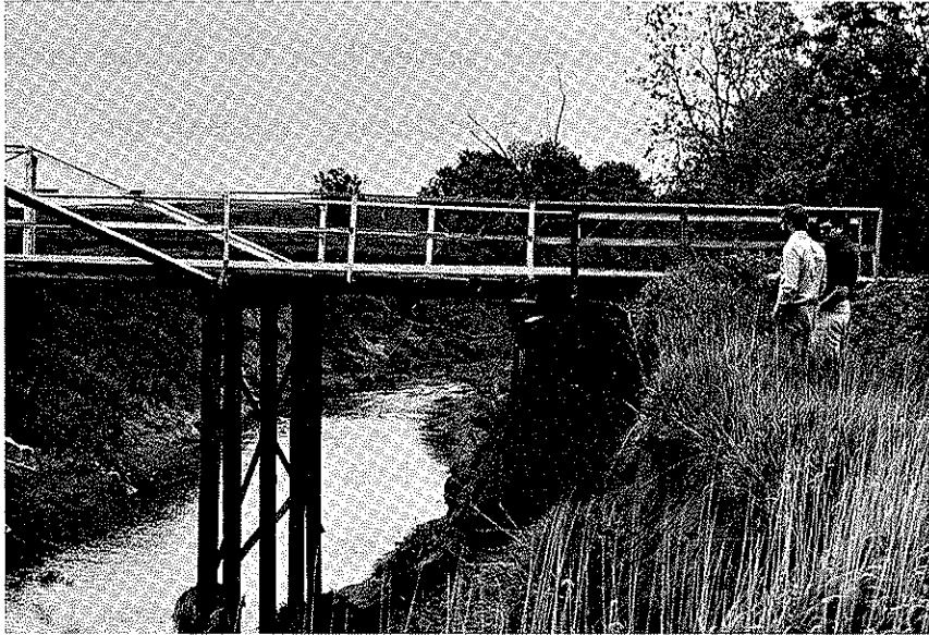
Plate 6. Stream degradation has exposed the bottom of the piles in this Crawford County bridge and caused a landslide which pulled soil from behind the abutment. Note that an approach span has been added to accommodate the increased valley width.
