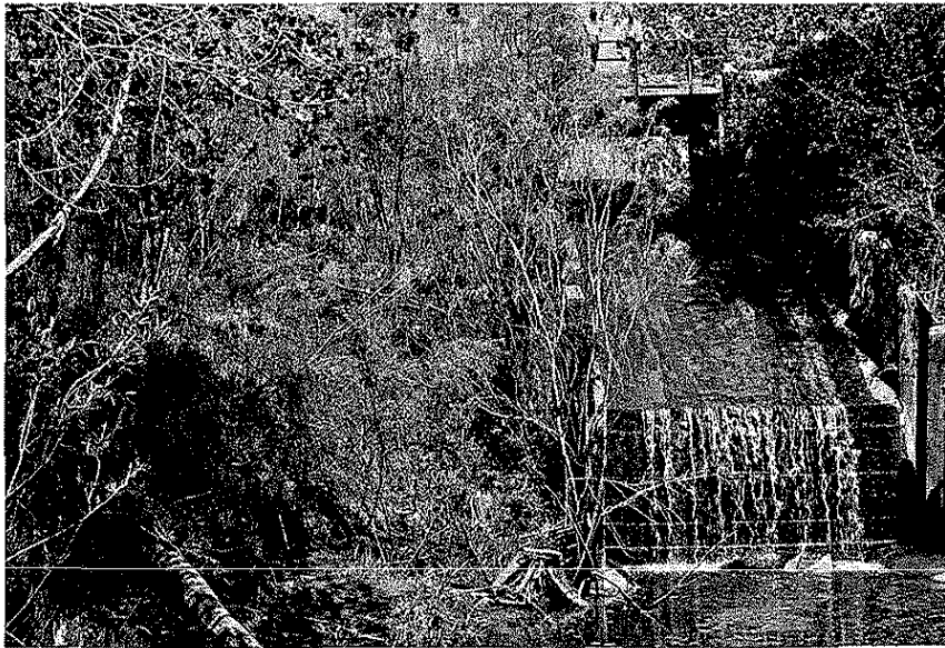
Plate 20. A foreshortened flume outlet; the irregular topography in the soil to the left of the flume is the result of landslides caused by seepage forces in the embankment.
