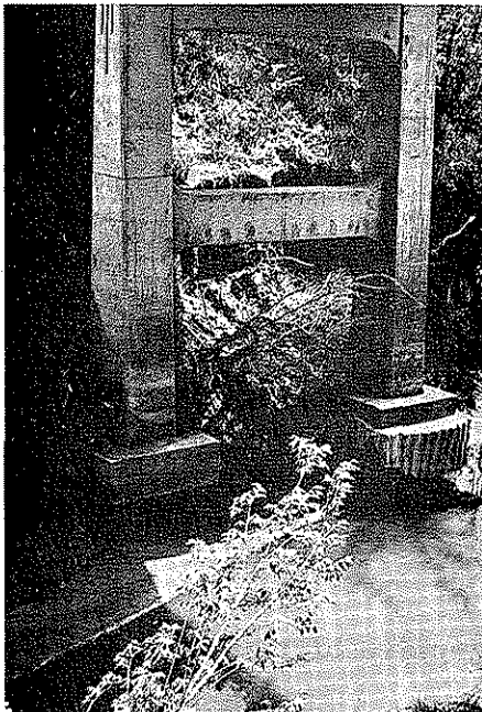
Plate 2. Degradation exposed pile cap of pier at left. Pier at right has had remedial work.
