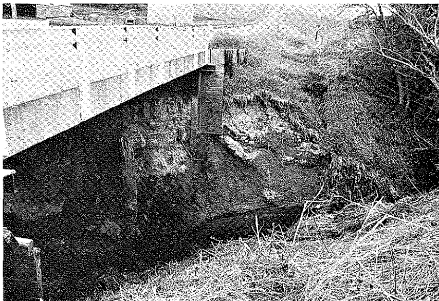
Plate 4. Degradation and the associated landslide has removed soil adjacent to the abutment on this Shelby County bridge.
