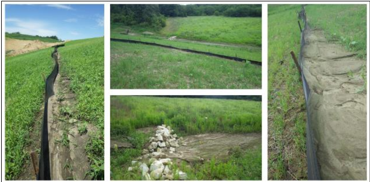
Figure 4. Erosion and sediment control devices at Mediapolis Site 1, including silt fences and a check dam
