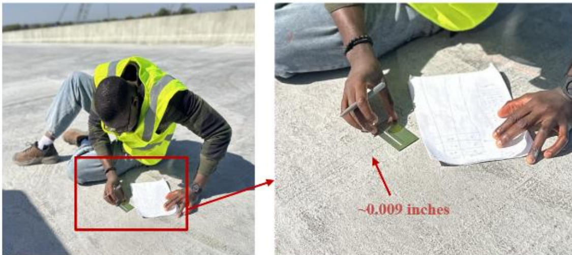
Figure 15. Ongoing measurement of observed hairline cracks
