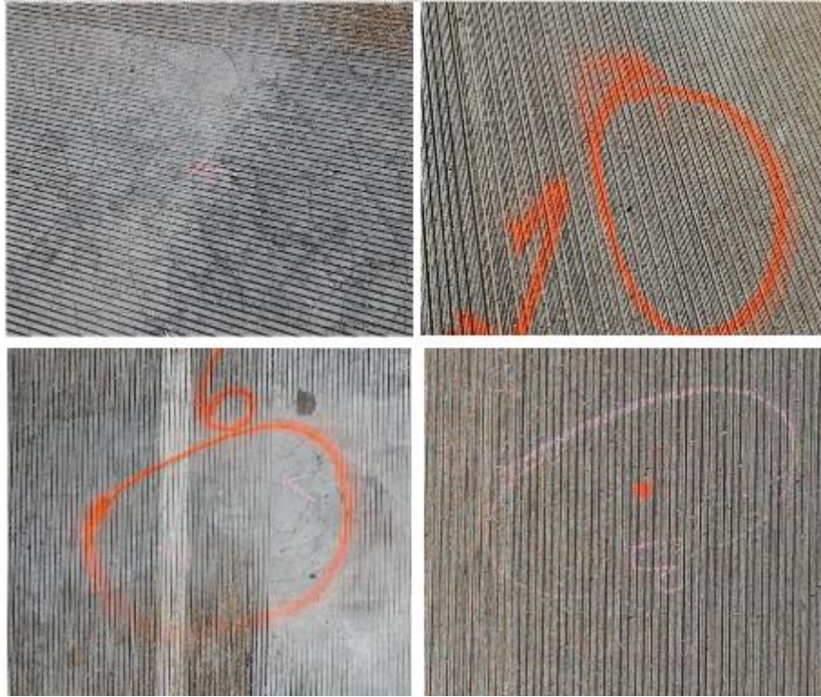
Figure 44. Identified and marked cracks on the bridge deck
