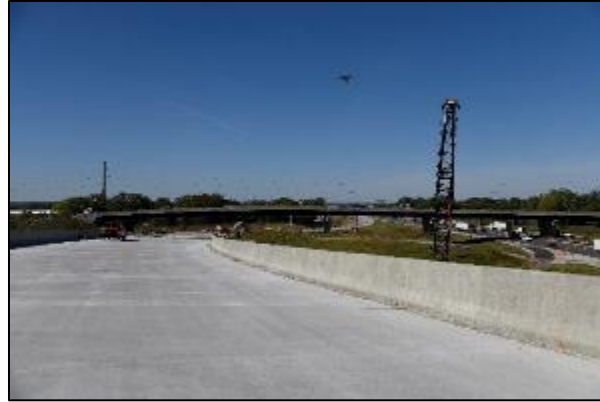
Figure 13. sUAS being navigated near the edge of the bridge to ensure that all target areas are covered precisely
