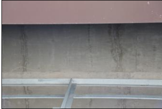
Figure 5. Cracks underneath the north side of the bridge
