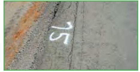
Required target density is not achieved
