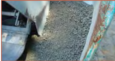
Segregation in paving hopper
