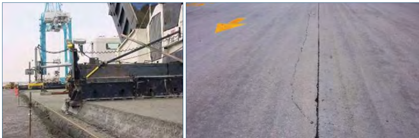
Figure 7-8. Paving shoe (left) used on the second lift, and longitudinal crack from first lift joint reflecting through adjacent second lane (right)
