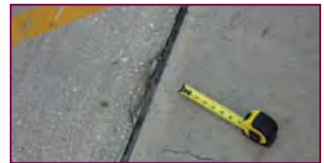
Spalling at cold joint
