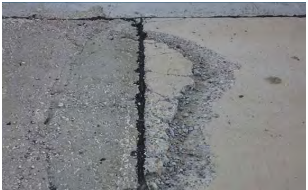
Figure 5-7. Distressed RCC possibly caused by expansion of the RCC slabs
