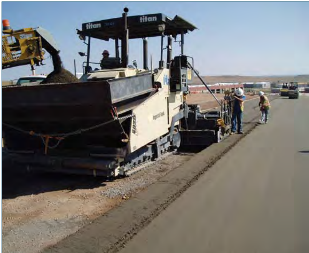
Figure 7-6. Fresh longitudinal joint
