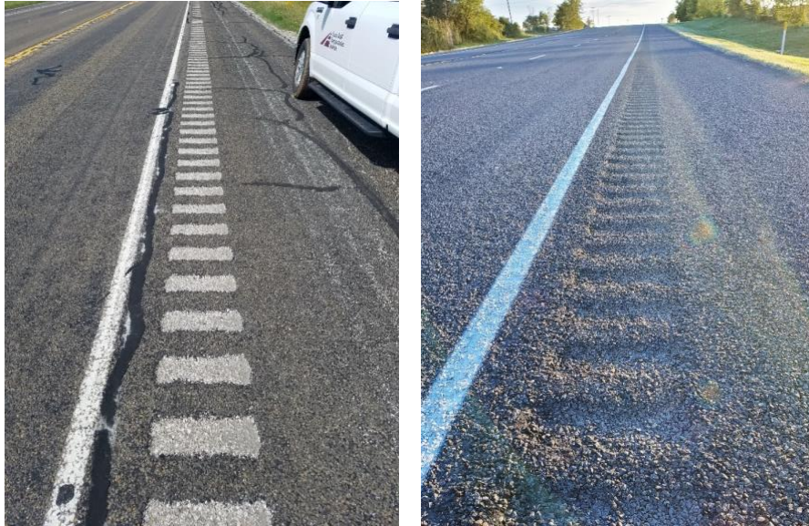
Figure 1. Rumble Strip before and after a Seal Coat Application.
