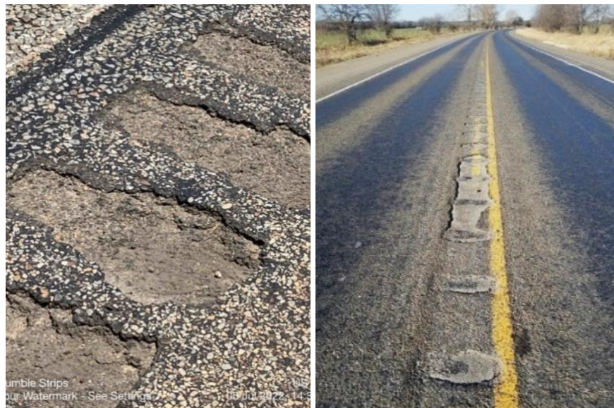
Figure 6. Rumble Strip Pavement Distress.
