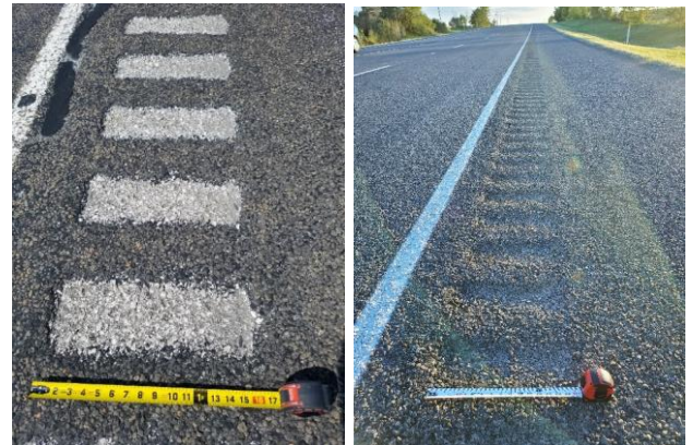
Figure 1. Rumble Strip Before and After Seal Coat.
