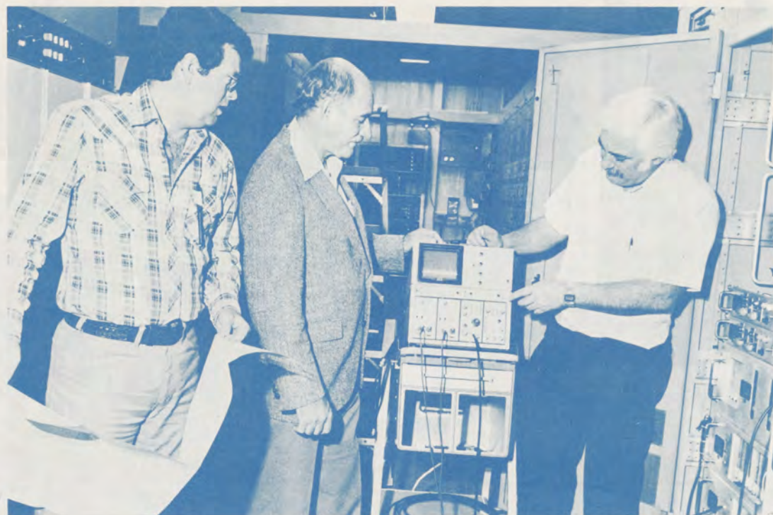
Top: Airway Facilities employees make adjustments on ARTS IIIA computer equipment. From left--Systems Performance Specialist Jordan Madison, Electronics Technician Don Hannum and Dave Lyons, ARTS Communications Unit Supervisor. (Photo by Bob Watson)
