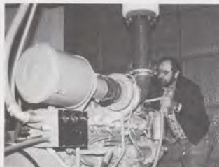
Environmental technician Charles Byrd makes a routine check of the tower's backup engine generator at the Raleigh Sector Field Office.
