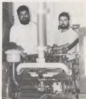
Electronics technicians Rick Marquez (left) and Jimmy Tarrant service the propane-fueled engine generator that provides backup power for the VORTAC.
