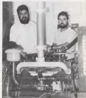
Electronics technicians Rick Marquez (left) and Jimmy Tarrant service the propane-fueled engine generator that provides backup power for the VORTAC.
