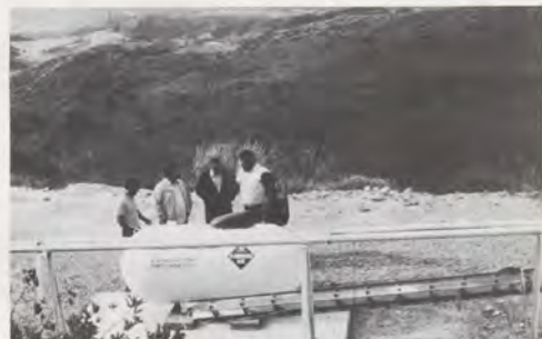
Los Angeles sector technicians discuss modifications that were needed on the new above-ground propane fuel tank that feeds the backup power generator.
