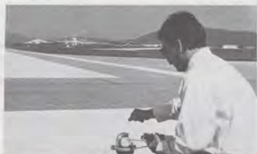
Threshold, runway edge, taxiway and obstruction lights are inspected to assure alignment, orientation and operation.
