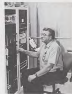
Los Angeles ARTCC systems engineer Ralph Danham gets the feel of the NARACS operating console in the center's control room.
