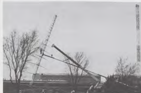
One can get some sense of scale of the global communications antenna about to be raised at the Los Angeles ARTCC from the figure of the technician half-way up.
