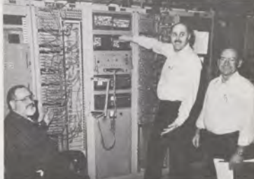
Inter-Facility Data Unit technician Joel Terwin (center) inspects new Back-Up Emergency Communications positions that were installed by Facilities & Equipment (F&E) technician Dean Bradford (left) and F&E supervisor Mel Maxey.
