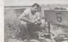
Checking transformers for the Runway 13L VASI Box is Environmental Support technician Bob Mazzara.
