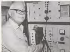
Checking the Andrews Air Force Base instrument landing system is Airway Facilities technician Evon Evans.
