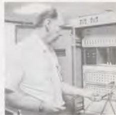
Ron Schultz, Kankakee assistant manager, patches into a second Model I communications line to bypass a line outage.
