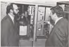
Looking over the ASR-9 transmitter at the manufacturing plant are Dennis Kolb (left) and Bill Restar.
