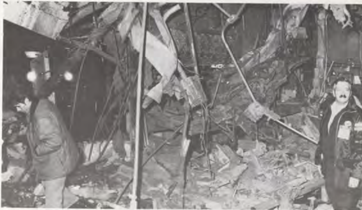
This locker area, the wall behind it and the ceiling above at LaGuardia Airport were blown apart by a bomb on Dec. 29, 1975.
