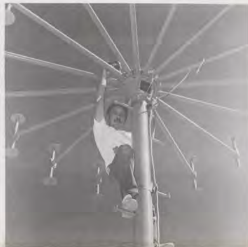
HANG TEN: Environmental Technician Sam Garcia of the Inyokern, Calif., Airway Facilities Sector Field Office shows why people in his line of work have to stay quick and nimble. What he's up to here (no pun intended) is installing an obstruction light atop one of the new solid-state Direction Finder (DF) antennas. Part of the Lancaster AF Sector, the Inyokern office is responsible for FAA facilities in 2,500 square miles of the Mojave Desert.
