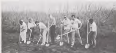
DIGGING IN: It's the ceremonial ground breaking for the new Maui tower in Hawaii. Construction of the $4.8 million structure now is underway and should be completed early in 1988. From the left are state airport manager John Sakamoto; Cheryl Peterson, Western-Pacific (AWP) Logistics; Danny Olivas, AWP Airway Facilities; Gordon Scrutton, Murphy Construction; Dick Thatcher, Maui AF Sector Field Office (SFO); Ken Brittain, project superintendent; and Noboru Nakao, Maui SFO.
