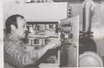
Electronics technician Paul Kessler, who works at the Louisville, Ky., Sector Field Office, does periodic maintenance on an engine generator control panel.
