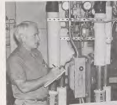
Maintenance mechanic James Barrett checks environmental controls at the Covington Sector's Lexington, Ky., AF Sector Field Office.
