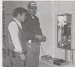
John E. Pope, supervisory engineering technician (left), and David L. Risinger, engineering technician, perform a Joint Acceptance Inspection on the power distribution for the Tandem System.
