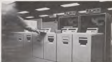
This bank of cartridge tape drives services the Host Computer. Easier and faster to load, it has more capacity and is 30 times faster in data transfer than the open-reel drives of the IBM 9020 computers.
