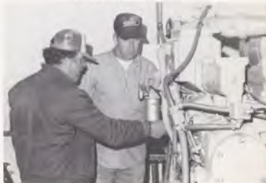
The Alexandria, La., long-range radar standby engine generator is serviced by maintenance mechanics John Duplisse (left) and Ed Walton.
