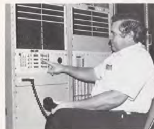
Working on integrated communications switching system equipment at DeRidder's Automated Flight Service Station is electronics technician Bill Kenney.
