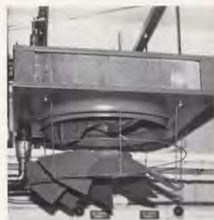
Part of the Pierce-Wohlford waste heat conversion is this heating coil fan unit attached to a cooling unit.
