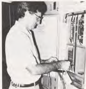
Maintenance technician Spiro Tsongalis tests circuitry in the equipment room of the Bridgeport FSS.
