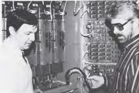
John Cotter, environmental systems engineer, and Bob Williams, environmental support technician, align the new power conditioning system for the Memphis airport's radar.
