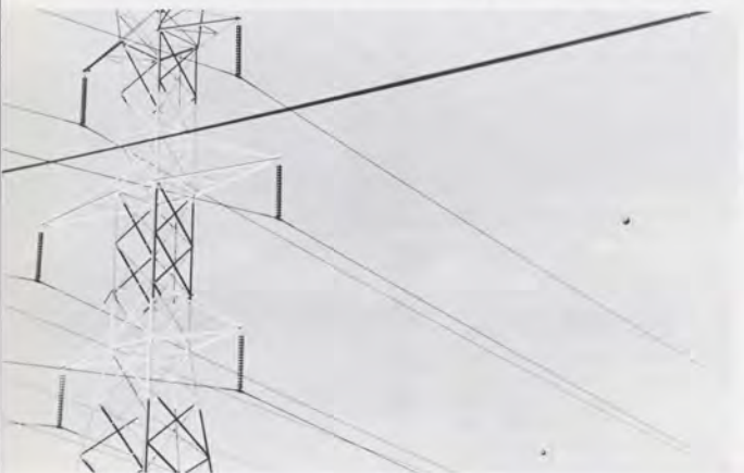
Orange globe markers are used to call pilots' attention to otherwise invisible high utility powerlines in the path of takeoffs and landings.
